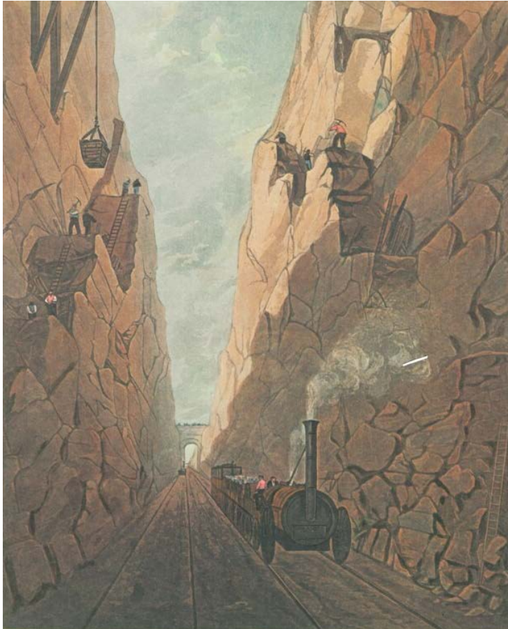
Top: The two-mile long, 40 feet high cutting at Olive Mount, still under construction in 1830.
