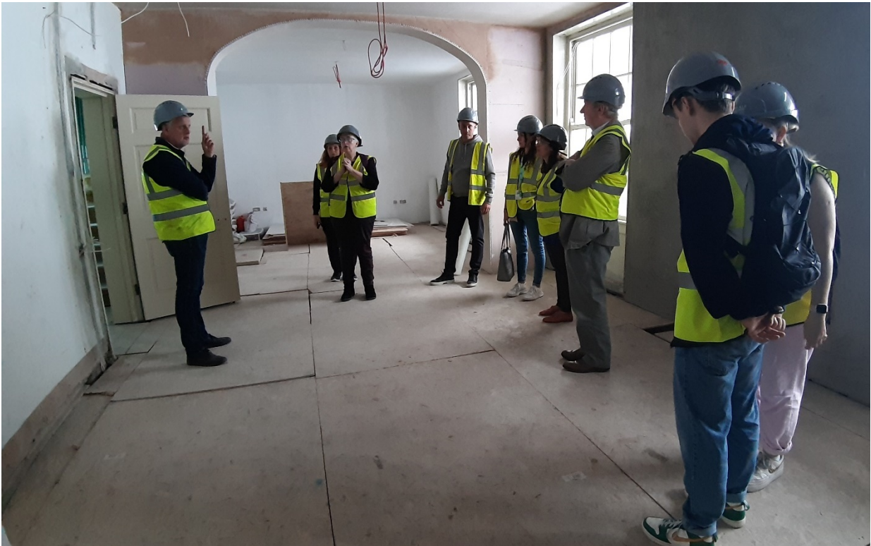
Visitors on a Scaffold Tour for Heritage Open Days in September 2023 getting a tour of progress on repairs to the roof and the first floor room, from Adrian Walker of Walker Construction.
