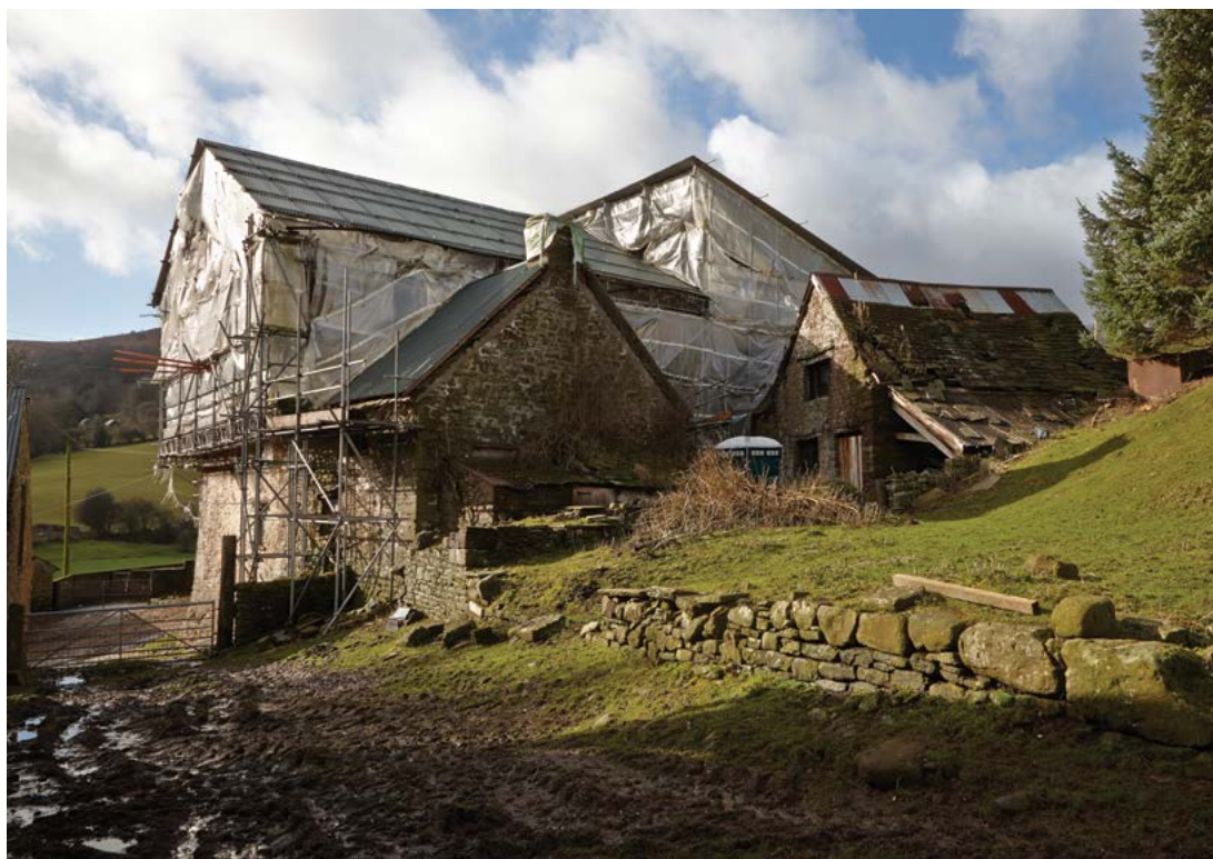
We are planning the rescue of Llwyn Celyn, one of the most important 'at risk' buildings in Wales.
