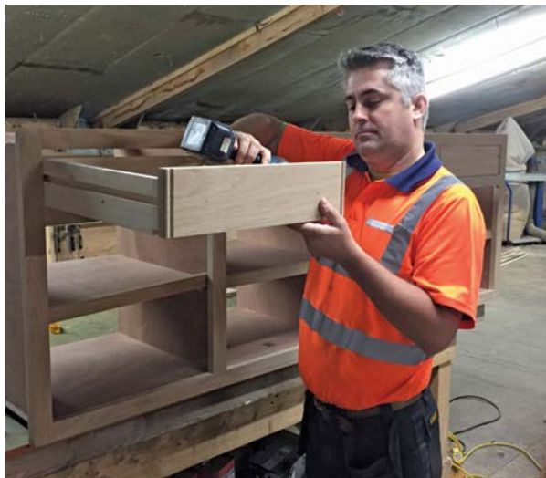
Marcin Sobczak building a new kitchen for Old Place of Monreith, Dumfries and Galloway.
