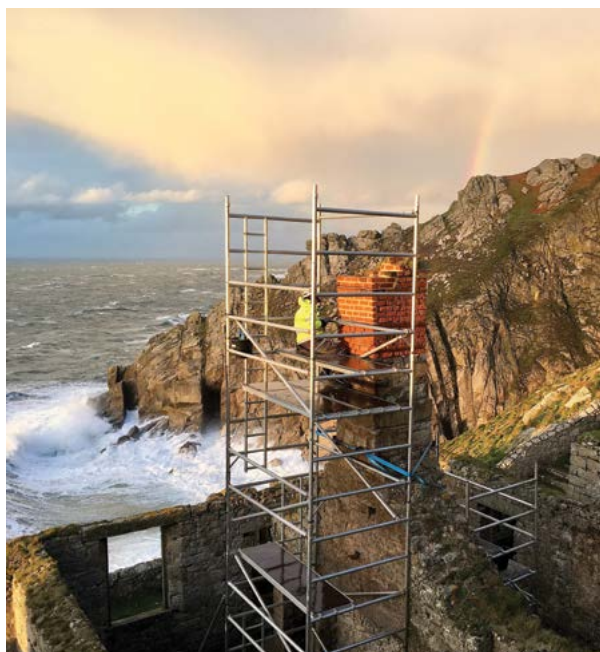
Stabilising the walls of the abandoned Fog Battery on Lundy to prevent further decay.
