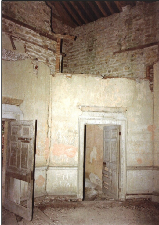
Destruction of the ceiling and cornice was almost total
