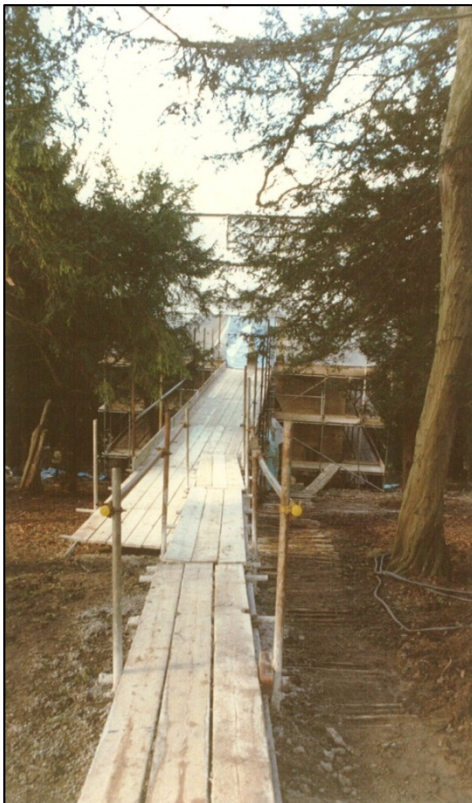
The slope down to the building became a morass of mud, so a walkway was constructed.
