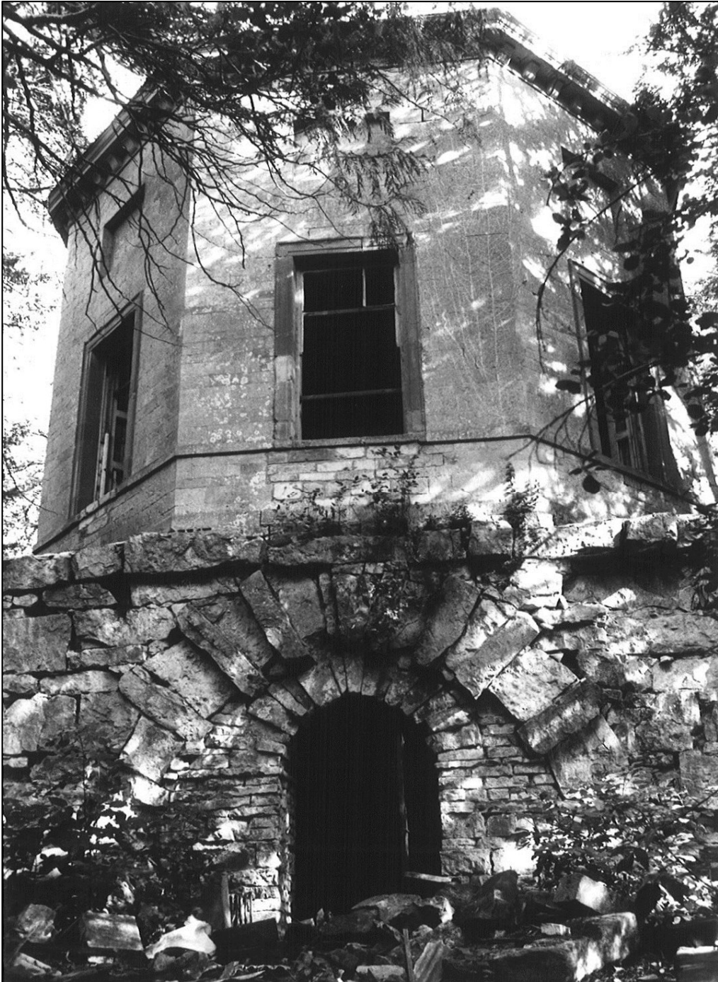
A photograph taken before the estate replaced the windows and repaired the roof in about 1970 after the most thorough campaign of destruction by vandals
