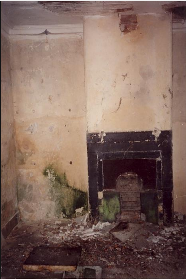
In the sitting room the cornice did not go round the chimney breast: perhaps the chimney breast was added later.
