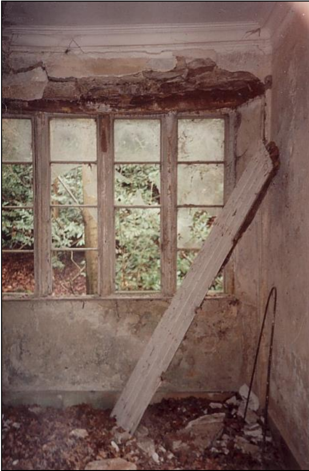
The sitting room, showing a rotten lintel above the north window.
