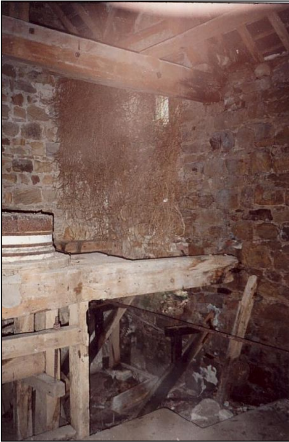
The beam in the south west corner in 1989. It had rotted below the damaged dormer window.
