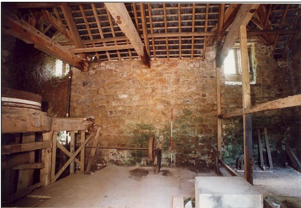
Looking west from the Mill door. The concrete blocks on the right, where the generator stood, have been removed.
