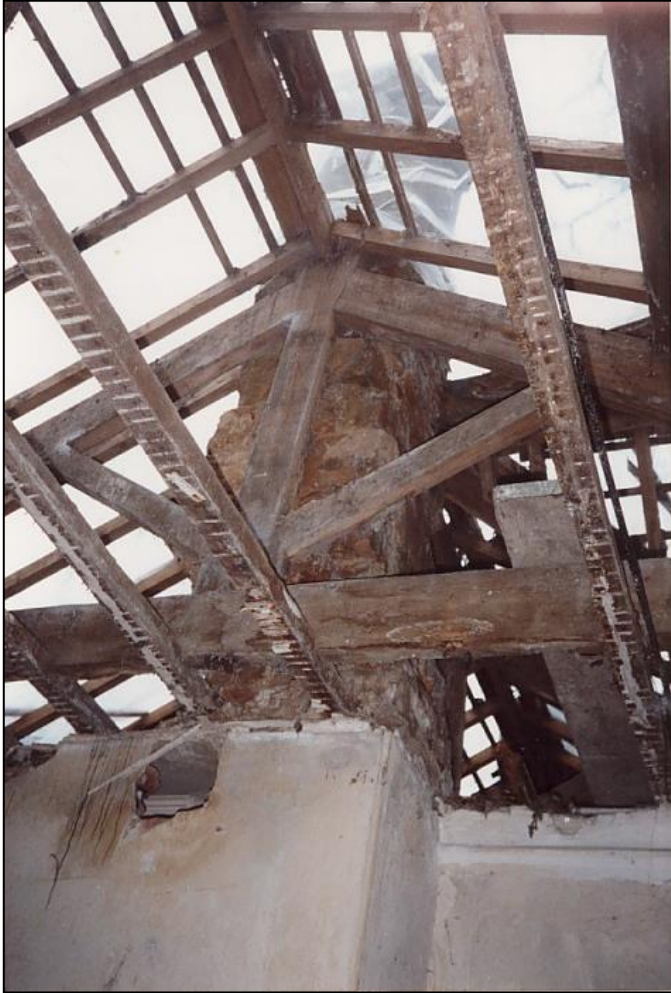
The sitting room chimney was frail and had to be rebuilt. The 19th-century truss is the same as the truss visible at the south end of the Mill, showing that in the 19th century the whole building was re-roofed at the same time.
