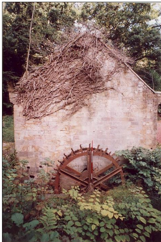
The south front. A blocked up slit window, under the ivy has been opened up.
