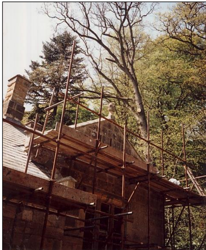
The sitting room chimney rebuilt. The acorn was found on the ground and was replaced on the gable.
