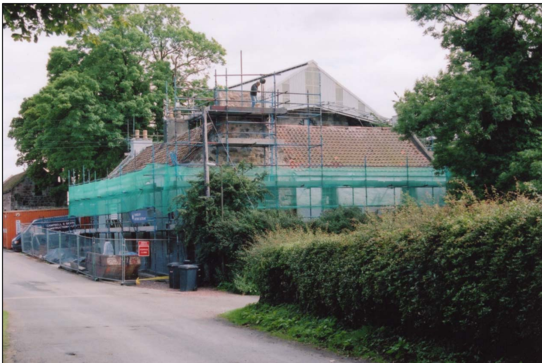
Work underway in July 2002. The temporary roof to Rosslyn Chapel can be seen in the background.
