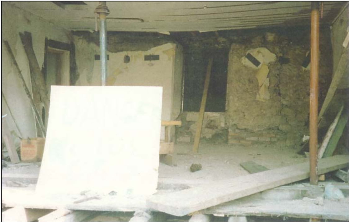
.Looking towards the street through the first floor bedroom at east end.
