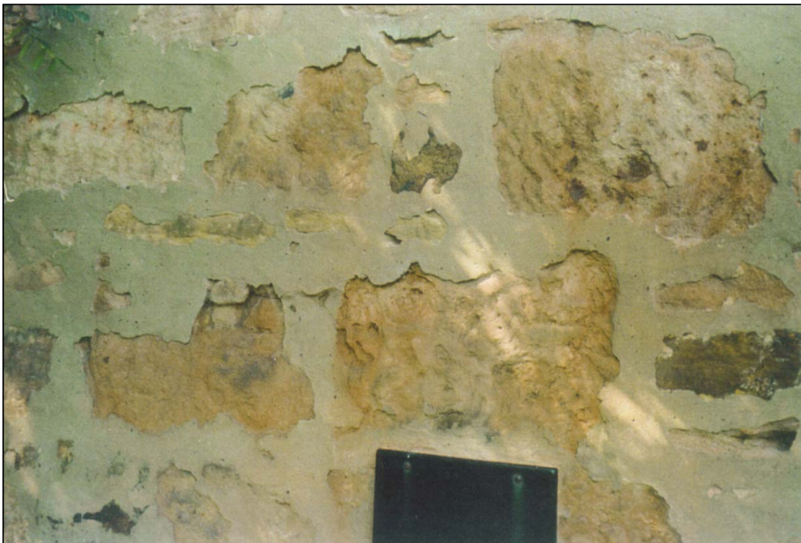
Poor pointing to the exterior of the south gable of the large sitting room prior to repointing
