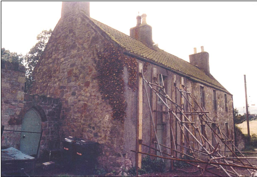
Not surprisingly, when the south wall of the east end collapsed in 1986, the whole of the east end was destabilised and the north wall had to be shored up.
