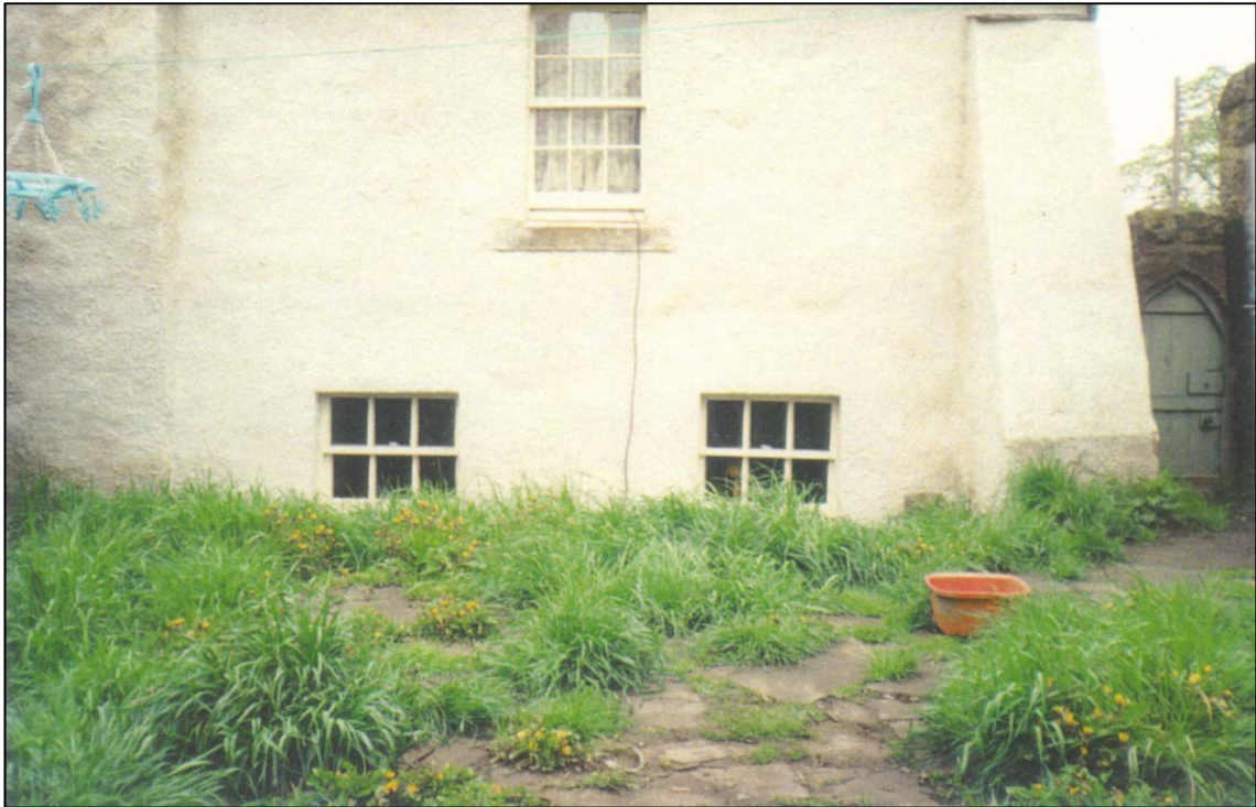
Ground levels at the rear had risen considerably over the years. In 1993 they were lowered by some 400mm shown here before the work.
