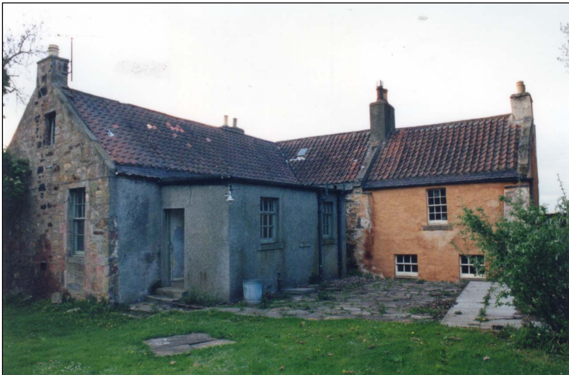
The building from the rear, before work began. The rather ugly kitchen and bathroom annex on the east elevation at the rear was then demolished.
