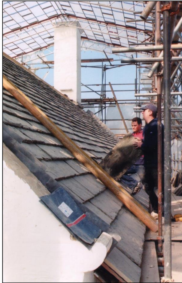
Fixing the stone rooftiles, huge at eaves level and representing some 35 tons in weight.
