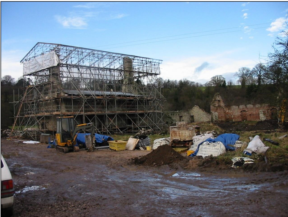
A canopy of scaffolding wrapped in polythene was erected to protect house and workmen from the elements.
