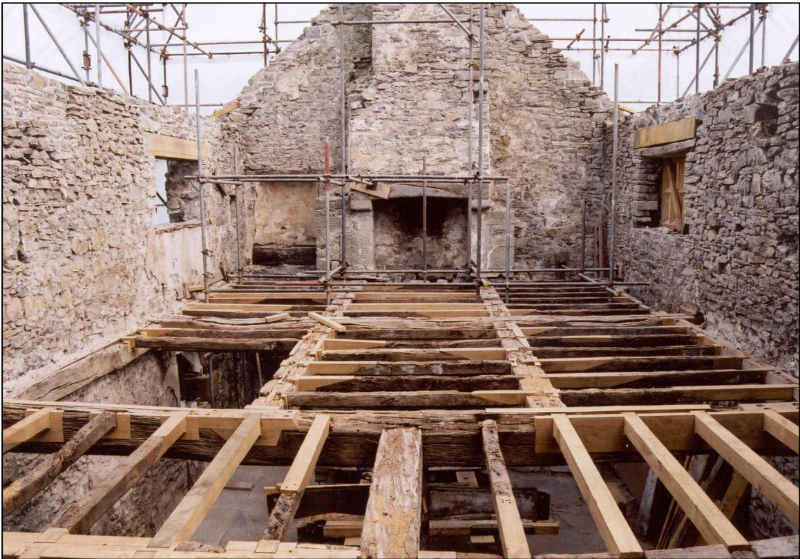
The first floor joists patched and reinstalled, looking across the solar floor.
