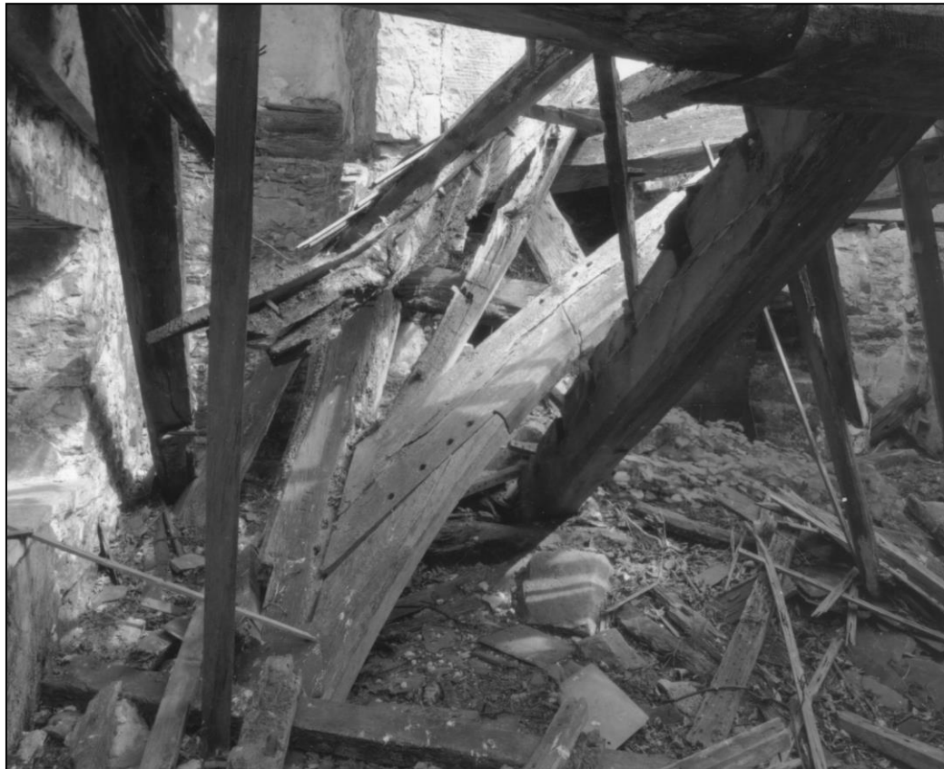
View north through hall, with collapsed arch brace from solar on floor.
