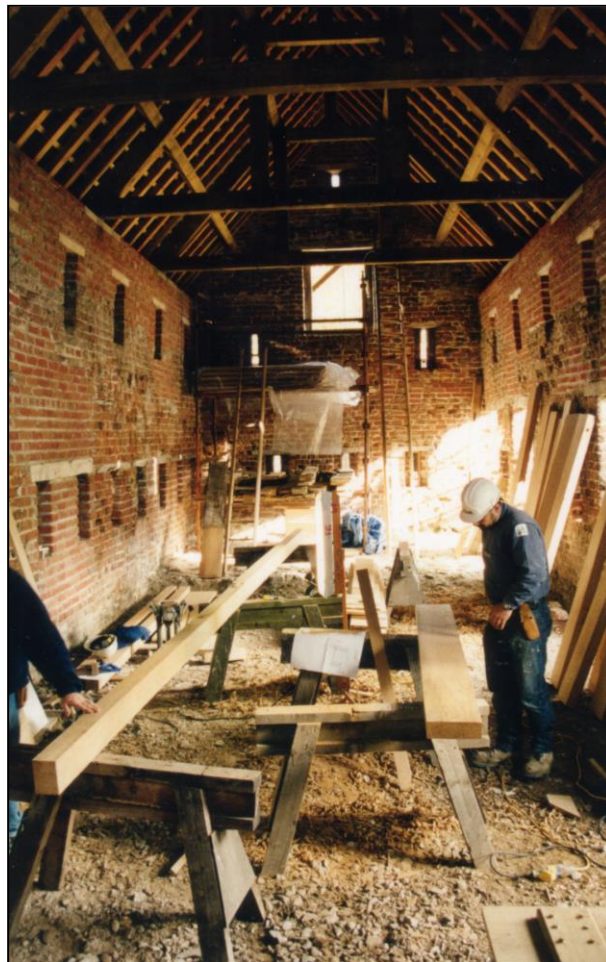
After repair with green oak, queen post roof at Cadw's request, the stables made the perfect setting out shed.
