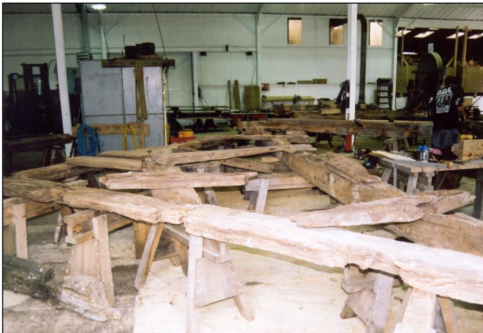
The arch-braced roof truss from the solar under repair at Carpenter Oak & Woodland's workshop in Perthshire.
