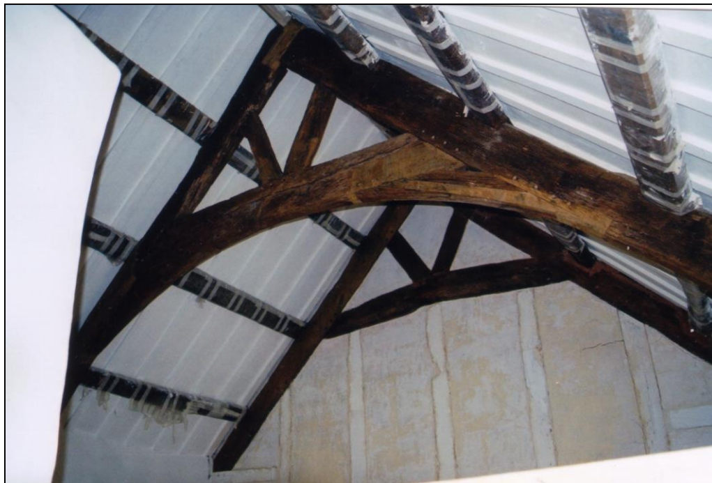
The solar ceiling: soffits torched and limewashed, purlins wrapped to keep them clean, screen partition limewashed, trusses as yet left clean. The roof is insulated with Cumbrian sheep wool (Cumbrian since Welsh sheep apparently have too oily a fleece!)
