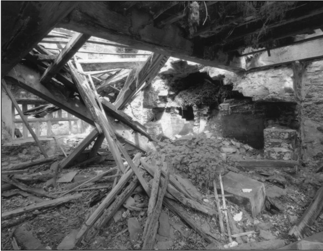
Hall fireplace – note removed bressumer under pile of rubble!
