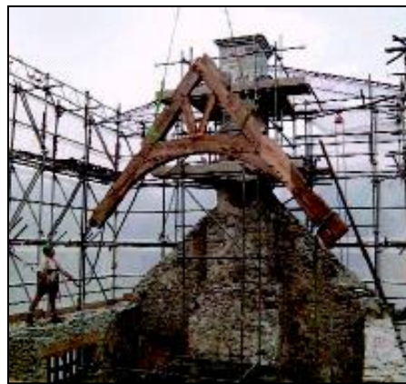
.... before being lowered back into place using a forty foot crane (July 2002).
