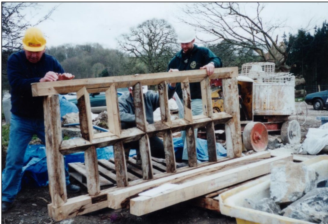
The east hall window repaired and ready for return to the building.
