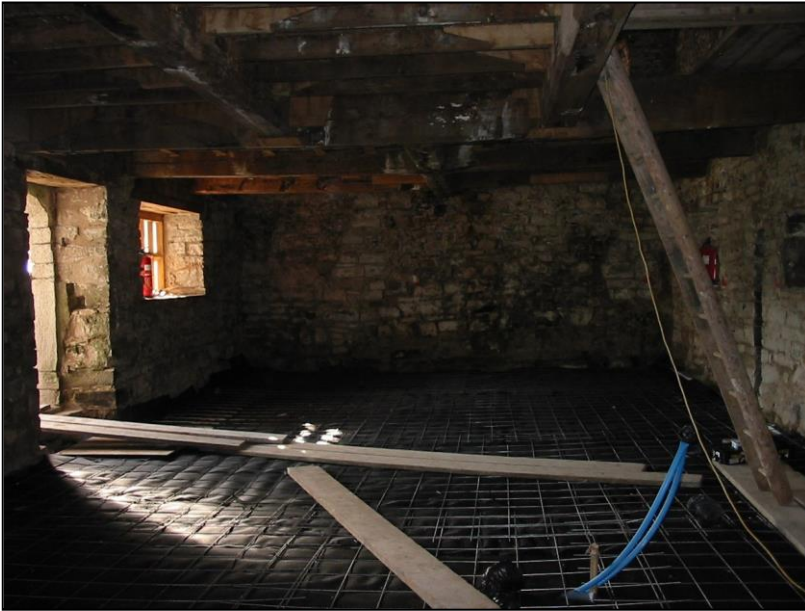
The ground floor cleared and the laying of the underfloor heating in progress
