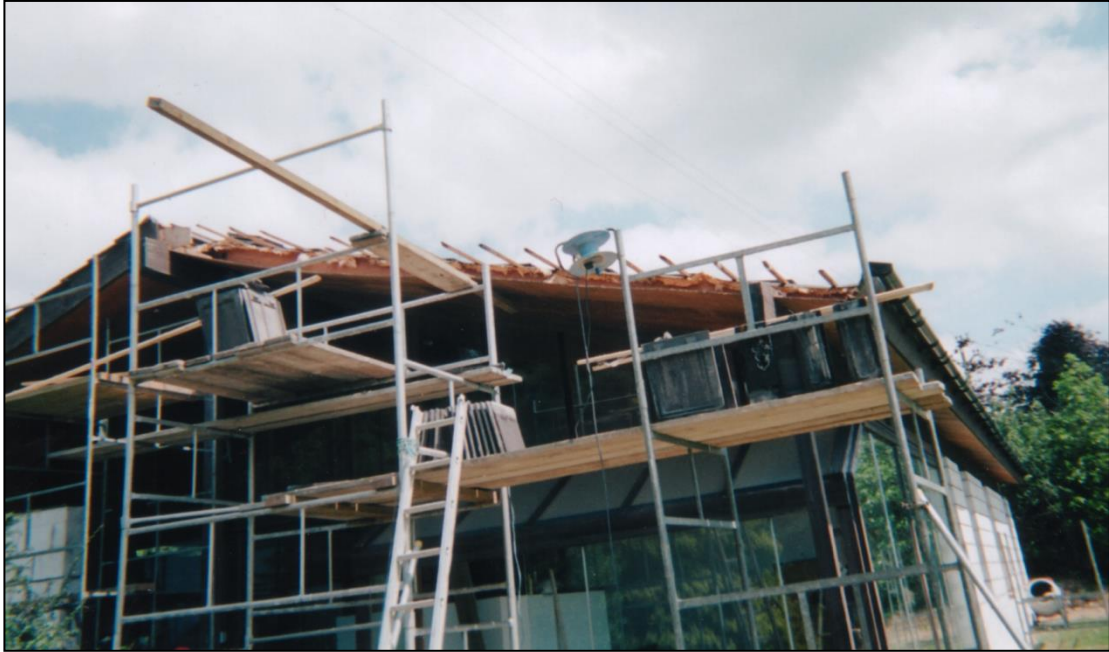
Water penetration had resulted in decay along the southwest corner at eaves level, which faces into the prevailing southwest wind. The roof was stripped back and battens and decayed timber replaced as necessary.
