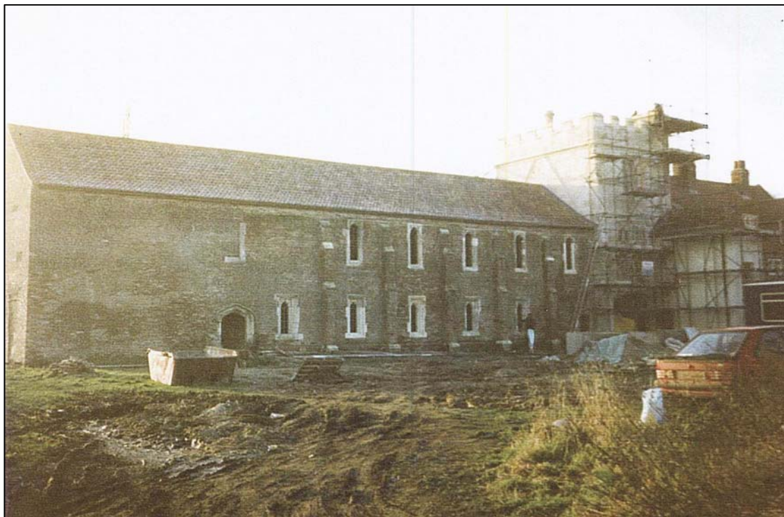
The window that was removed to make the barn opening was restored
