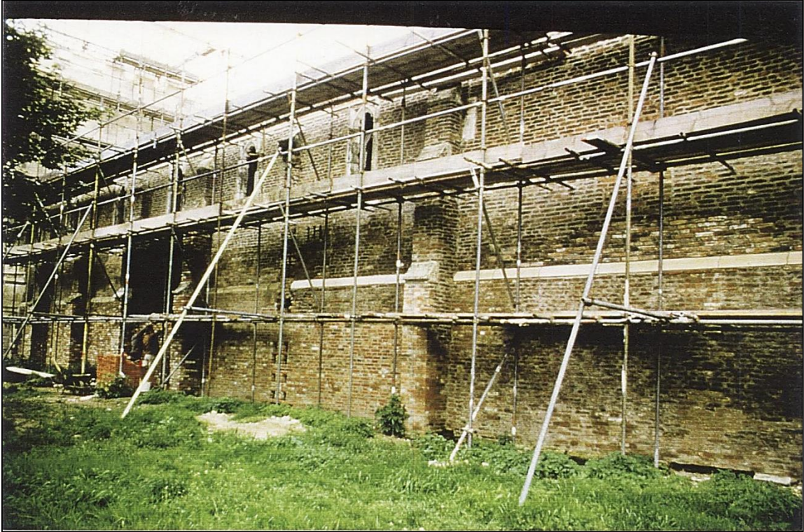
The barn door being bricked up on the south side; one buttress is still missing
