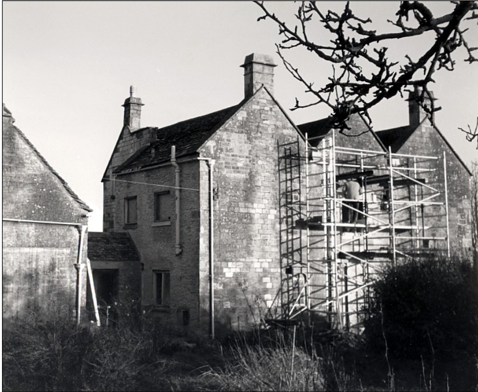
Work on the west front, with a new door and window added.
