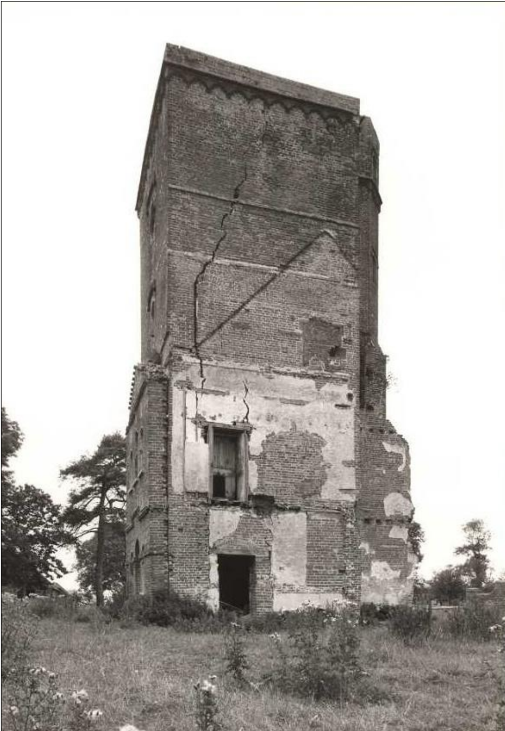
The North East Face. The remains of the 18 th century additions can be seen in the gap between the pediment and the face of the tower.
