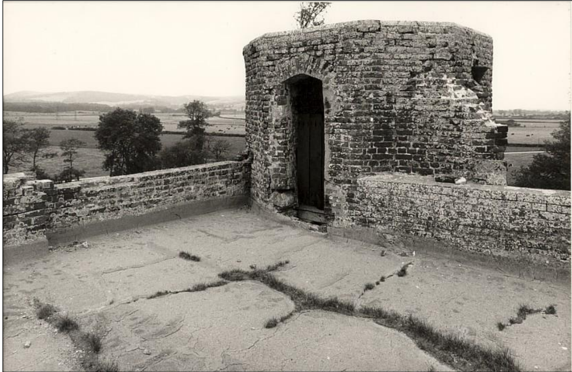
The Roof. The tower had been given a new roof during the War to make it safe for use as an observation post. This probably saved it from total collapse in the following decades, but by 1978 it was itself in poor condition.
