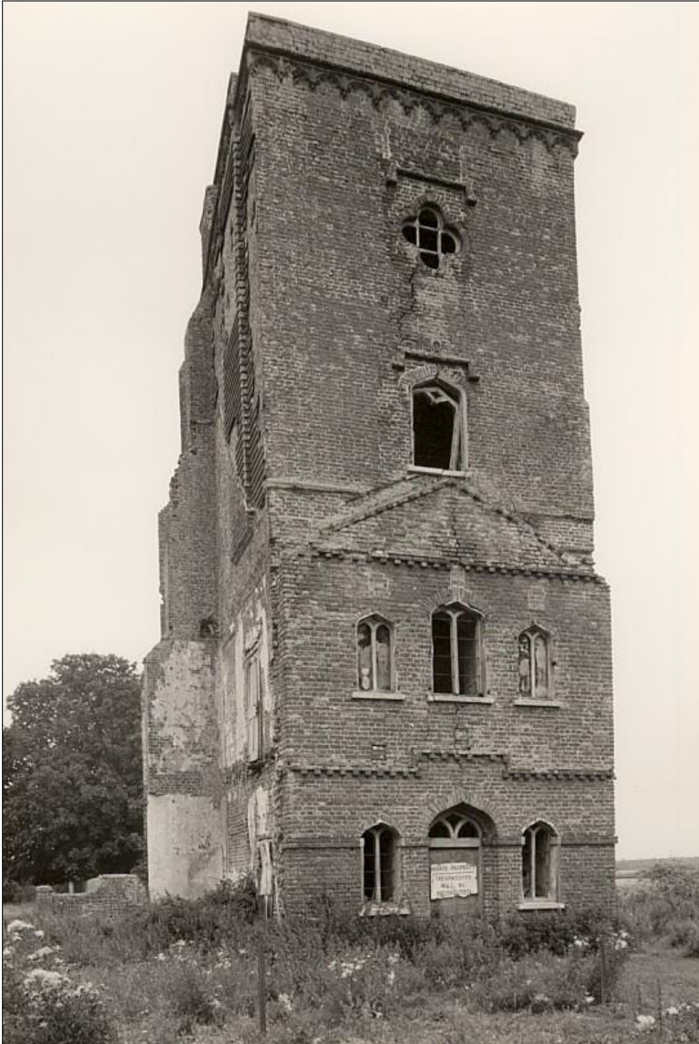
The South East Face. The front wall was bulging outwards, forcing the brickwork of the pediment away from the face of the tower, and allowing water in behind. The door and window joinery was in a better state than it looked, and could mostly be
