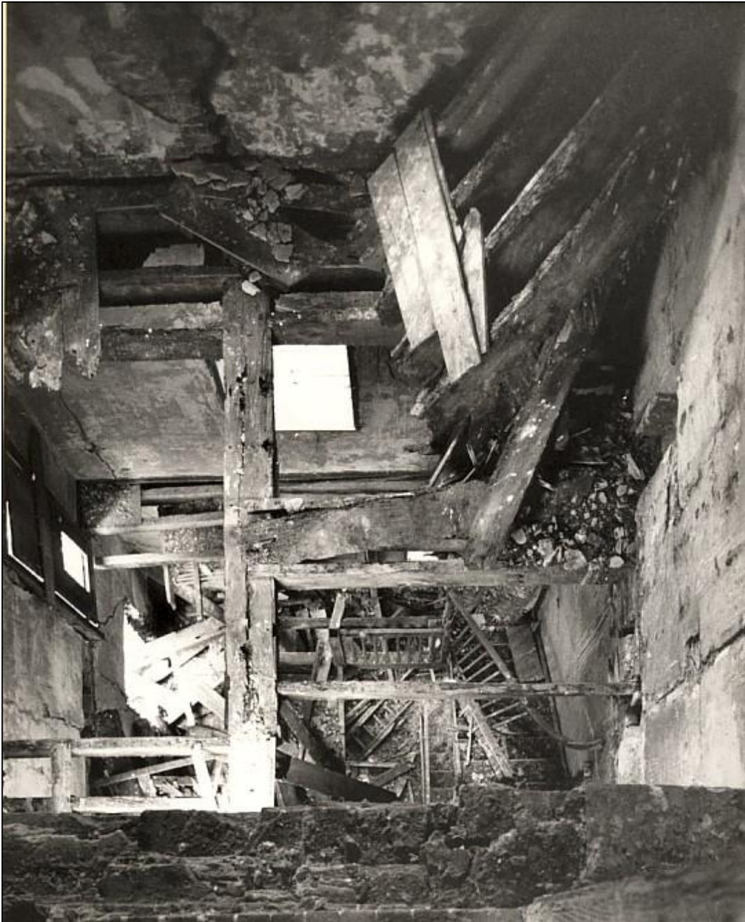
Inside the Tower. This photograph was taken from the door opening into the third floor room from the stair turret. Surprisingly, a number of the floor beams and joists were sound enough to salvage for reuse. Under each floor now is a grid of steel ties holding the four walls of the tower in place.
