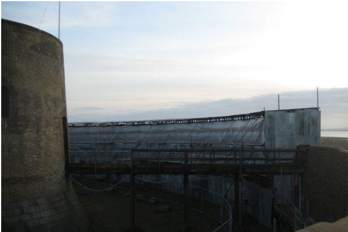
The glacis walls, scaffolded and sheeted against the elements for lime work in 2020-21.
