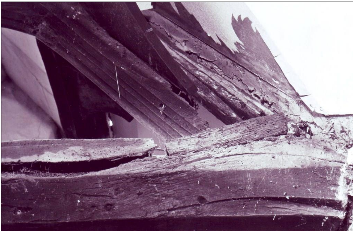
Decayed ends of main truss timbers.
