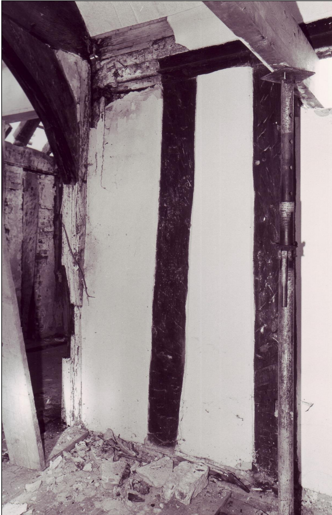
As the later plaster was removed, the moulded timber cornice was revealed.
