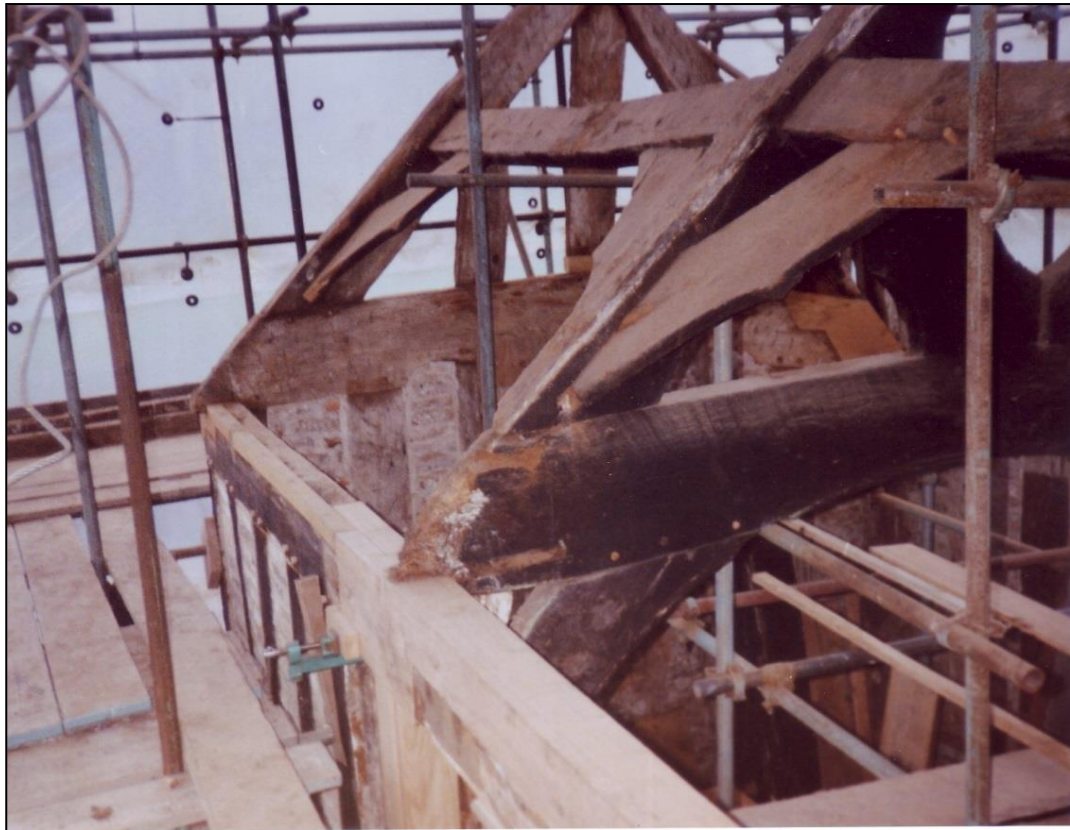
Architect Andrew Thomas inspecting repairs to the roof timbers (in blue coat, top picture).
