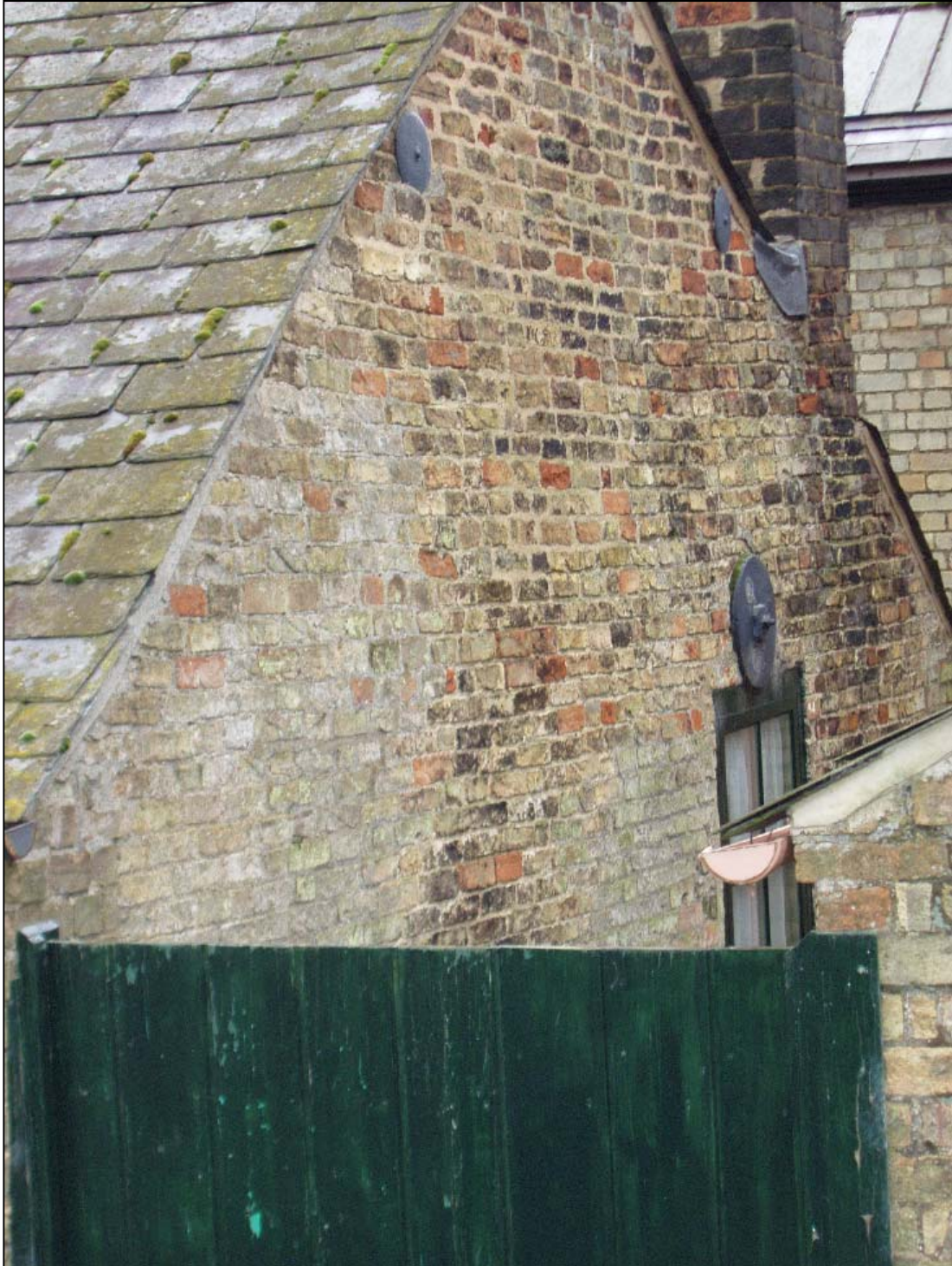
The re-used bricks from the earlier windmill on the site are clearly apparent in this end gable.
