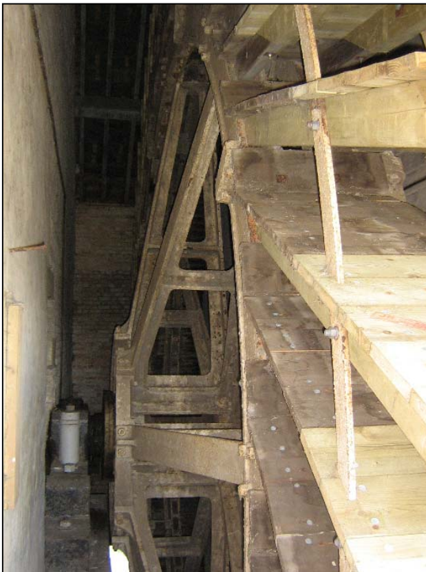
The surviving scoopwheel, installed in 1896. Today, levels have shrunk so much that its paddles would barely reach the surface of the water, if the drain still remained.
