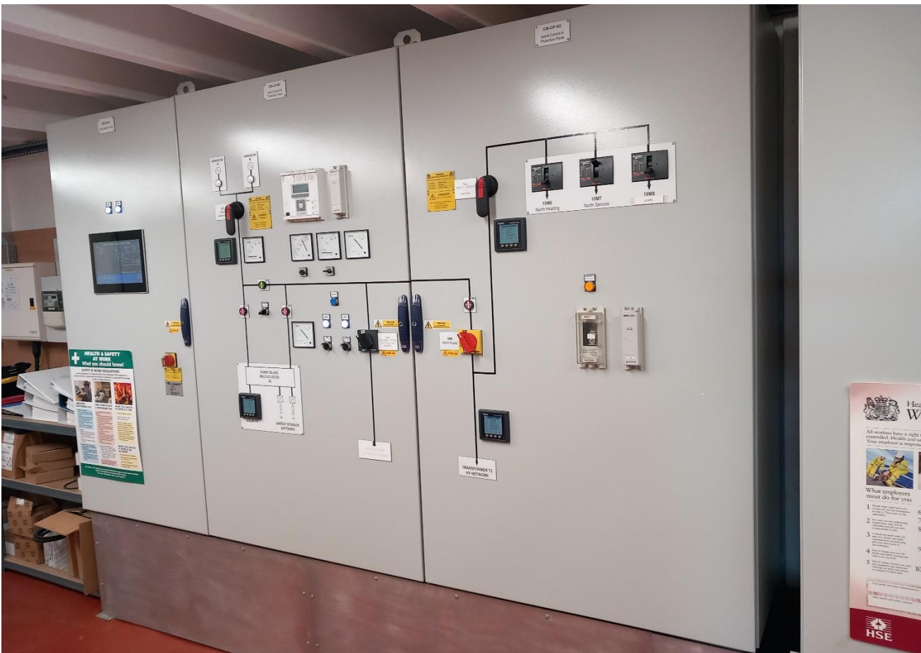
Main control panel
