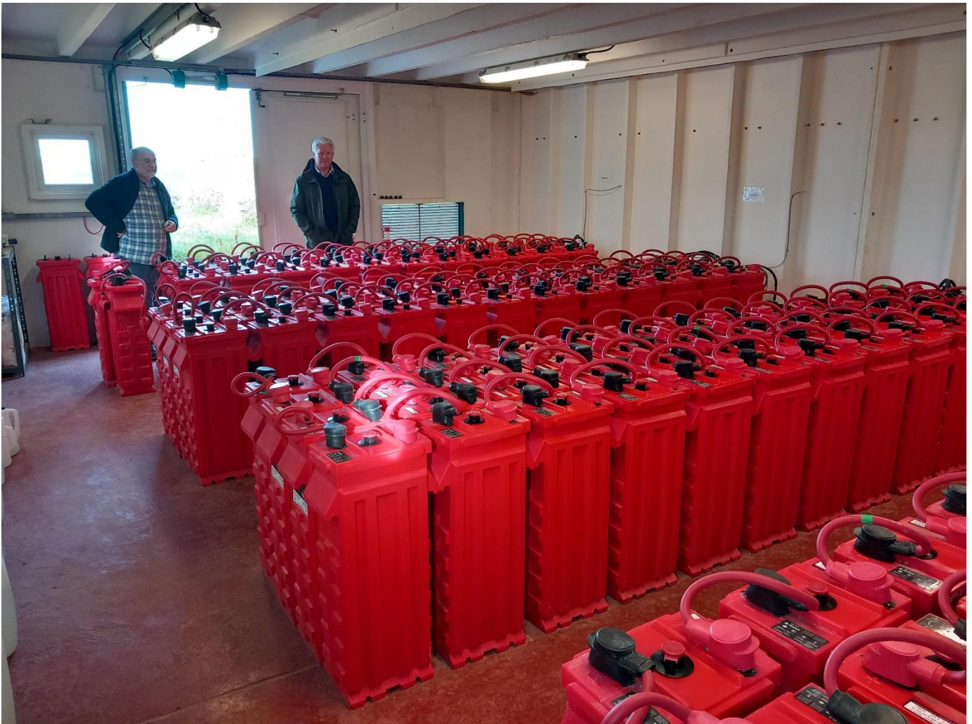
DC Battery clusters – Each “bank” contains 48 individual batteries
