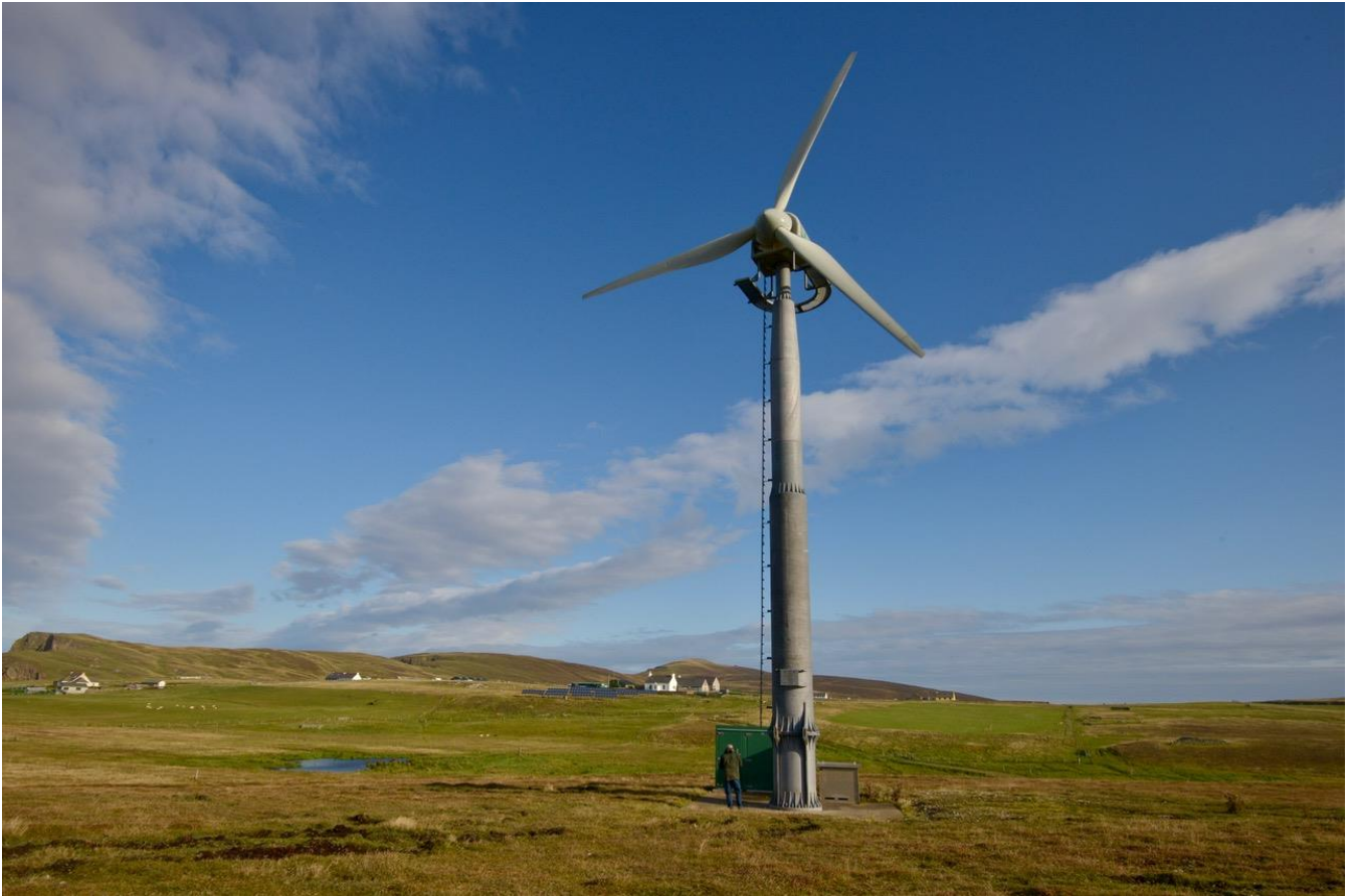
Harbon 60Kw Turbine
