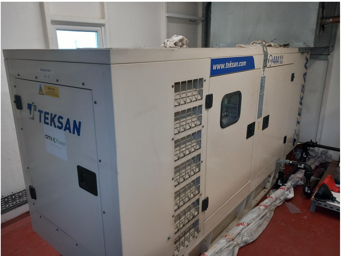
80Kw Acoustically clad Generator
