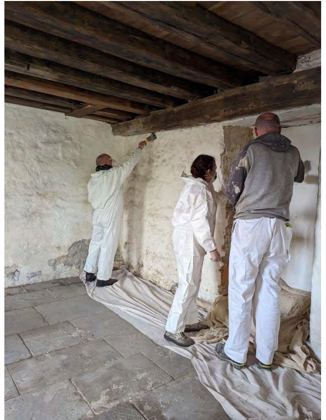
Volunteers learnt about limewash and then used it to redecorate the chapel walls.
