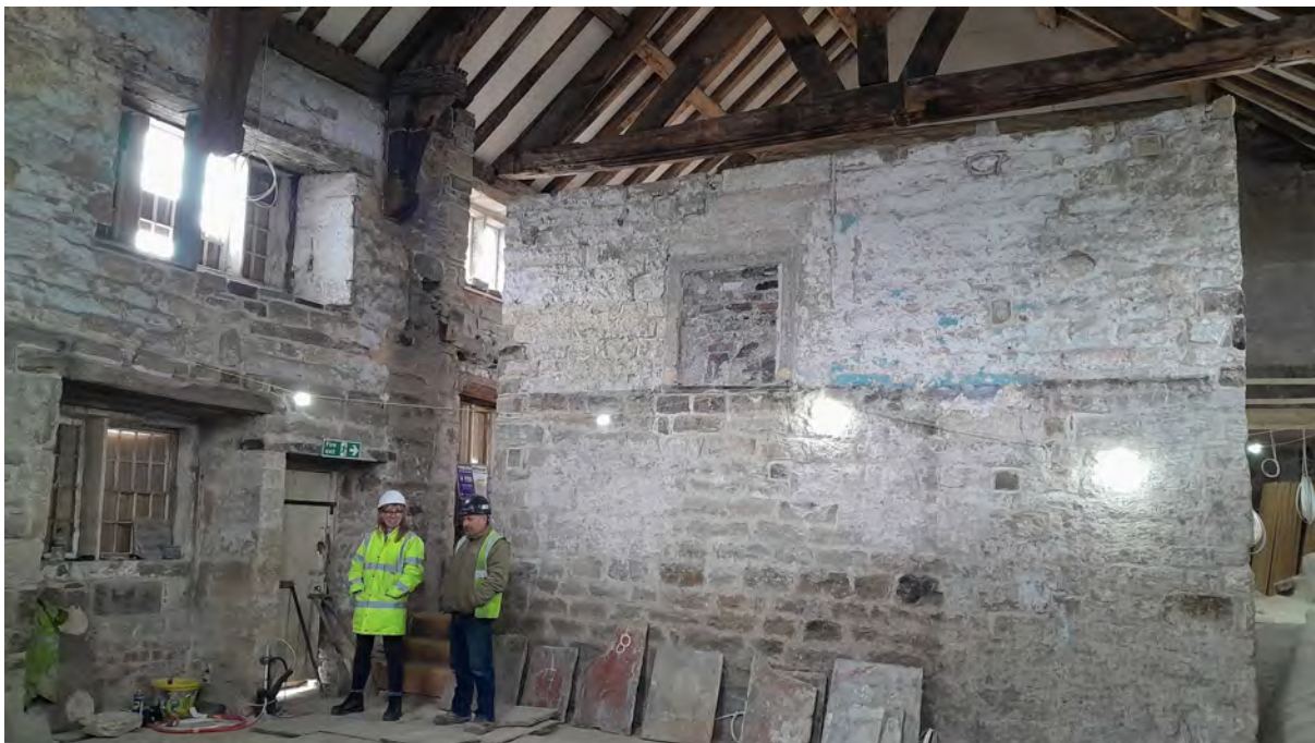
Linda Lockett and Andy Dewhurst contemplate the challenge of installing the panelling in the Great Hall. The image top right shows how far out of true the southeast wall was.
