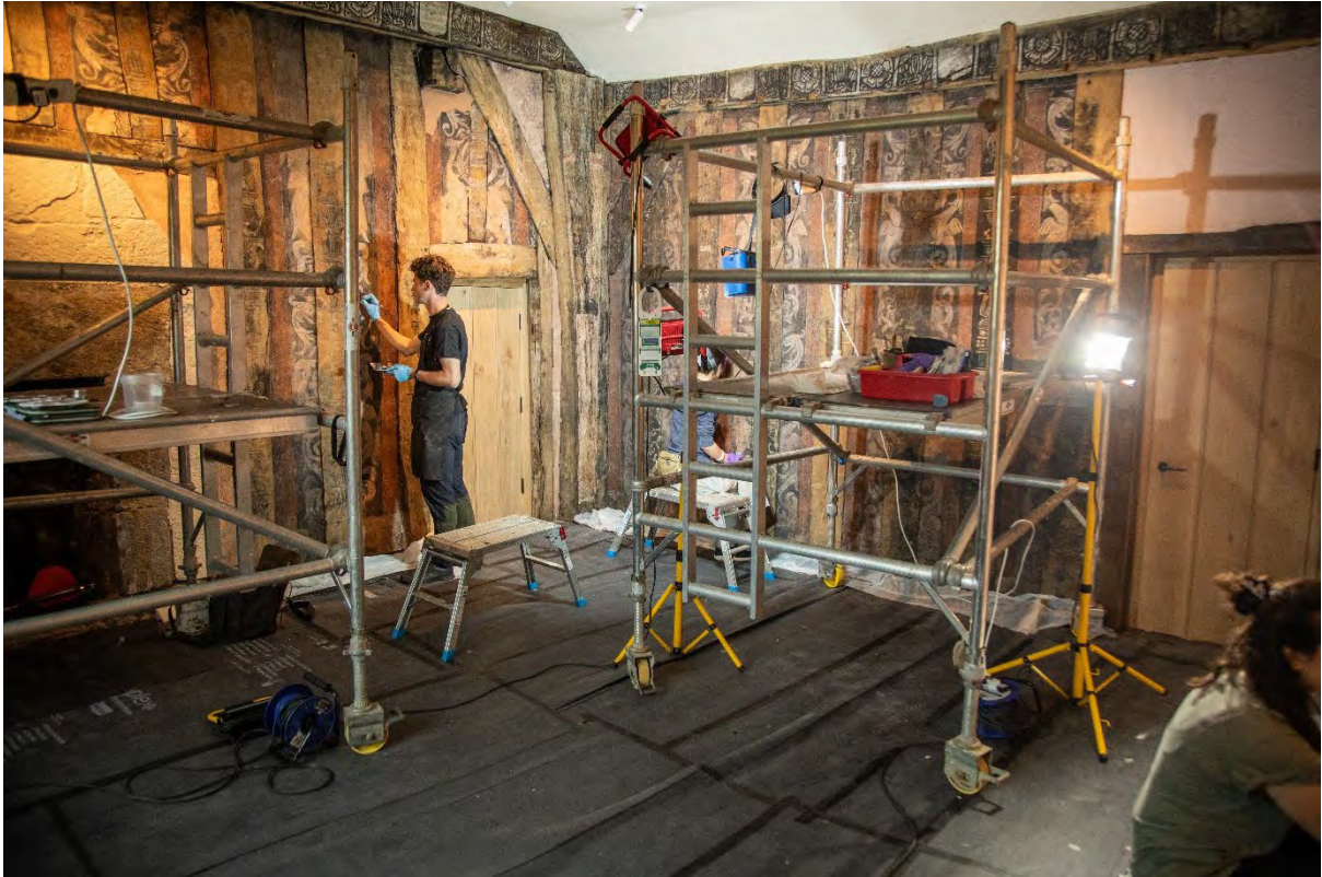
Top: the northwest wall as first revealed. Below: conservation work under way by Opus Conservation in summer 2024.
