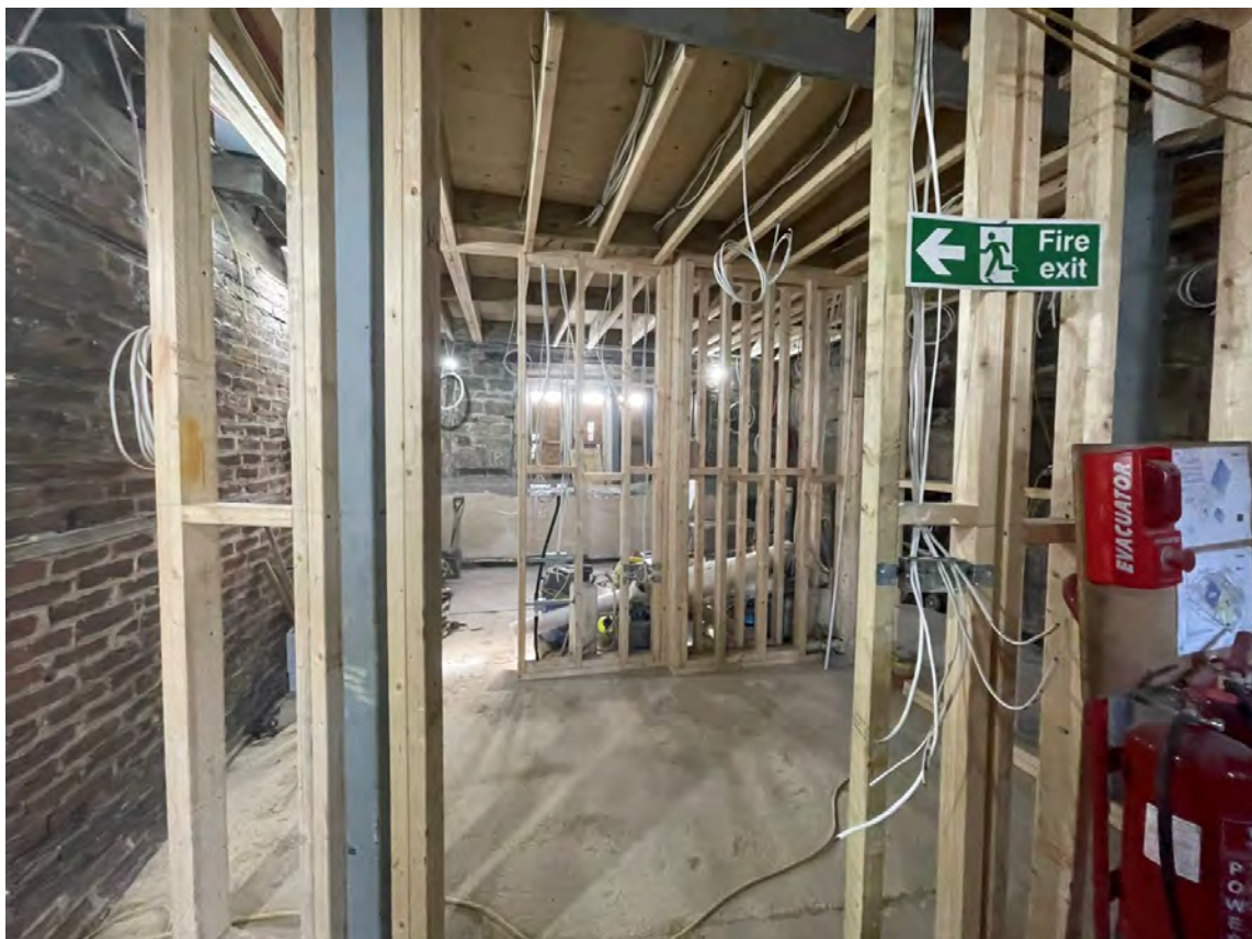
A forest of wires and timber partitions, precursors to the creation of the bedrooms and bathrooms on the ground floor of the Solar Block. Such use echoes the service rooms that occupied the ground floor originally.
