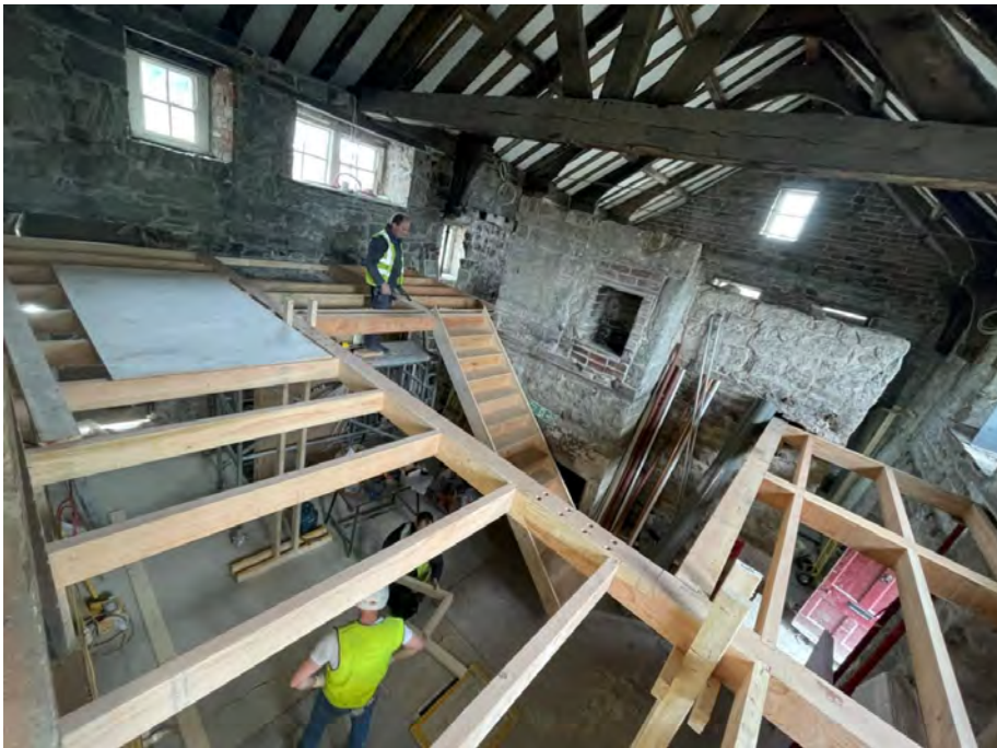
Constructing the mezzanine floor. A temporary ladder stair was in place for much of the project. The late-17 th century partition wall has been reduced in height, cleaned off and repointed.
