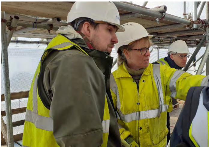
Landmark's senior surveyor, Linda Lockett, discusses a structural point with structural engineer Robert Ratcliffe.
