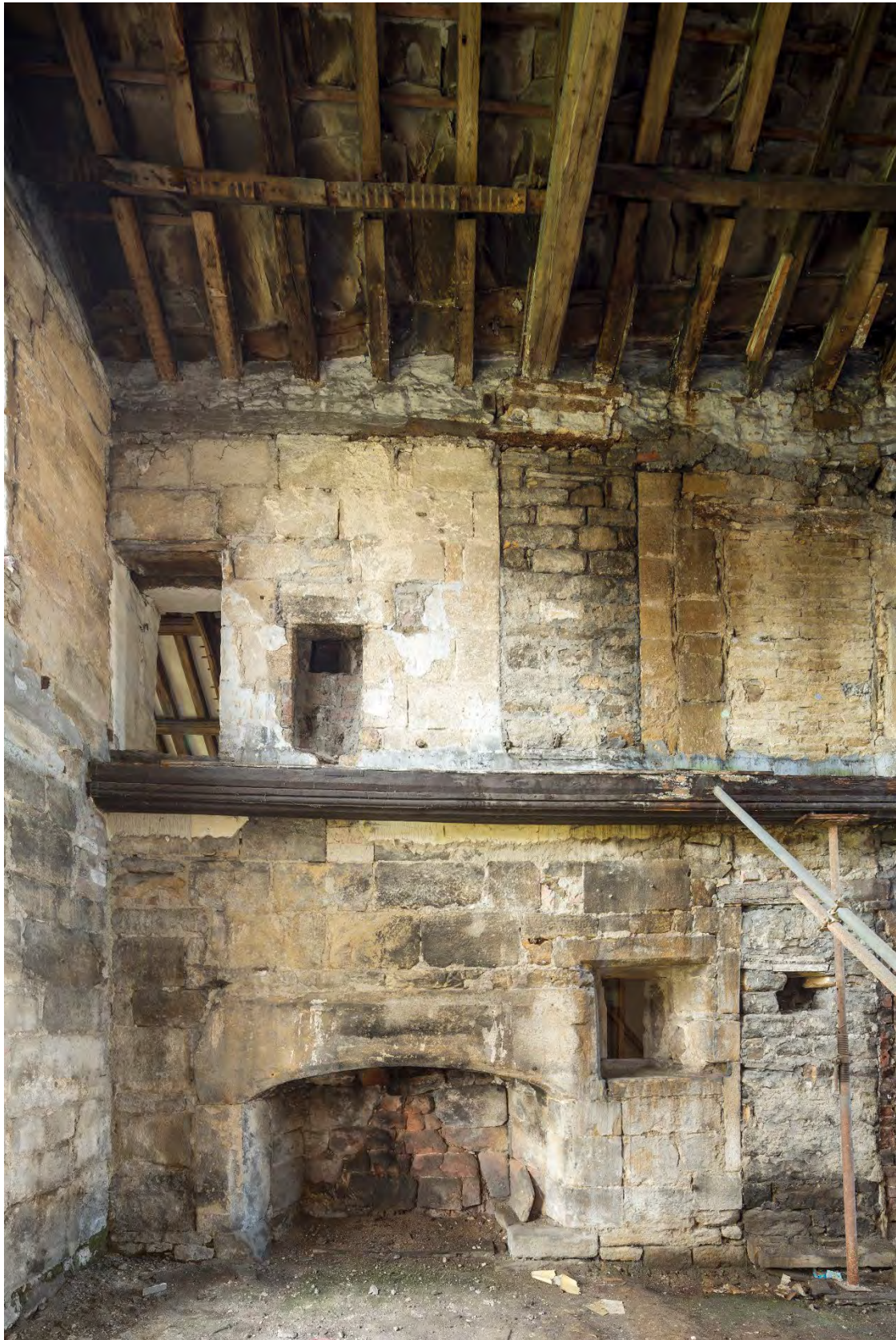
The much-altered southwest end of the Solar Block in 2020, extended in the 16 th century and with a glimpse of the Chapel gallery roof through the doorway
