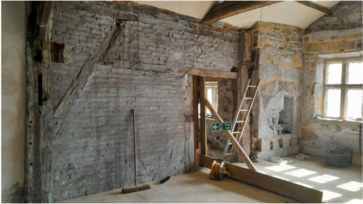
Residual framing from the 1320s hall block, and the original doorway into the first-floor hall, now in use once more, after raising the lintel to take account of modern statures.
