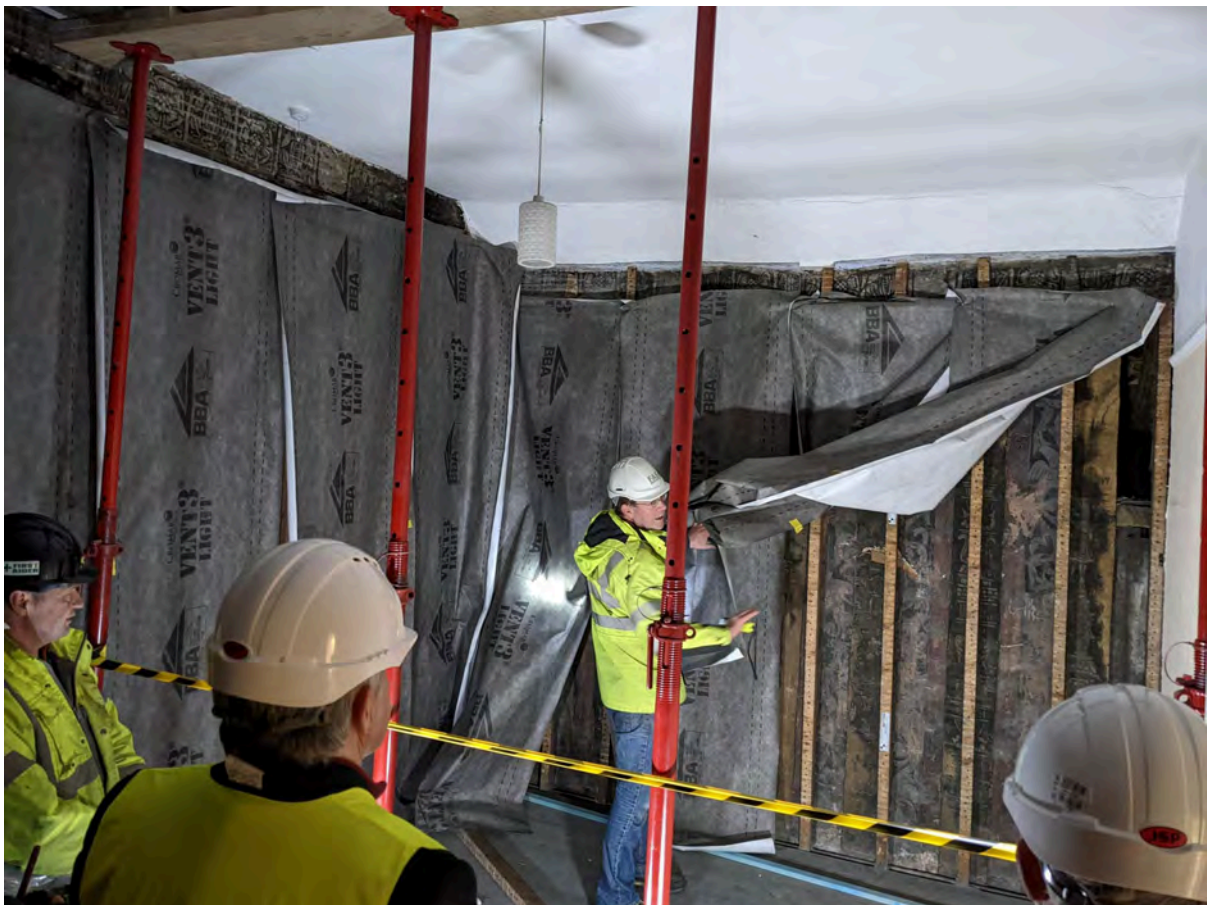
With permission to remove the lath and plaster walls, but the supporting stud work still in place for now, for a couple of years the wall paintings were carefully protected, later with Perspex sheets, revealed only occasionally.
