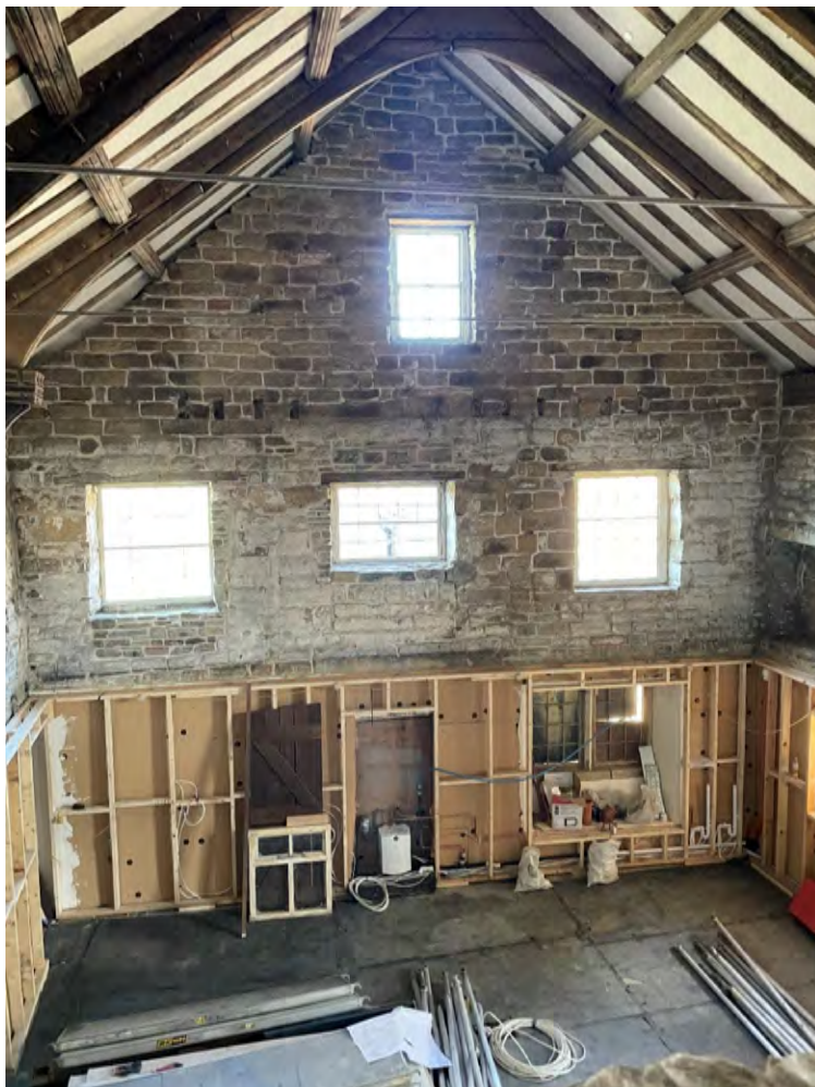
The framework in place for the panelling. The finished panelling provides additional insulation as well as holding pipework for the kitchen and electrical ducting, and being aesthetically pleasing by drawing the space together.
