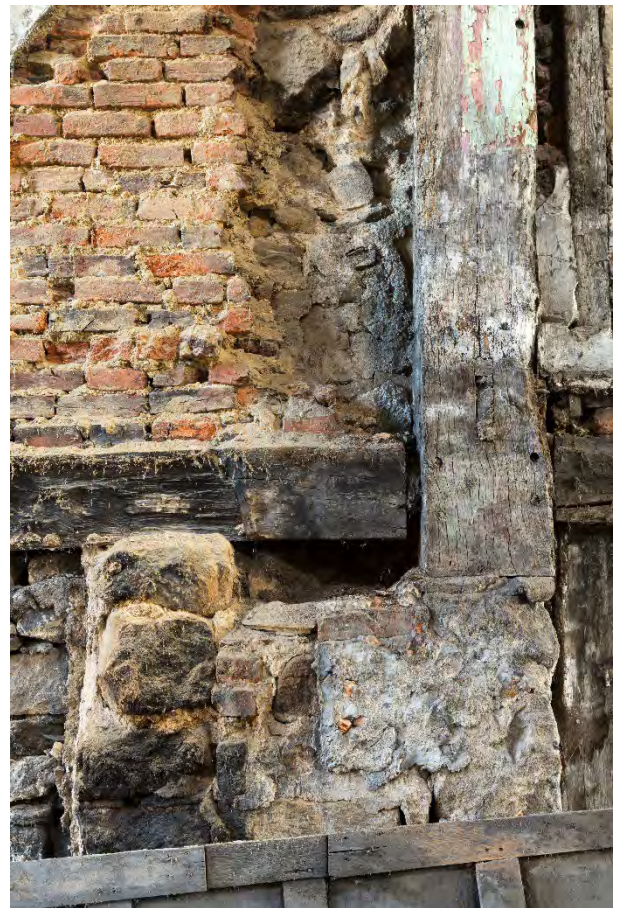
A post from the early 1320s hall house that survives as part of the structure of the Solar Block. The early hall is thought to have had a stone ground floor with a mostly timber-framed first storey.
