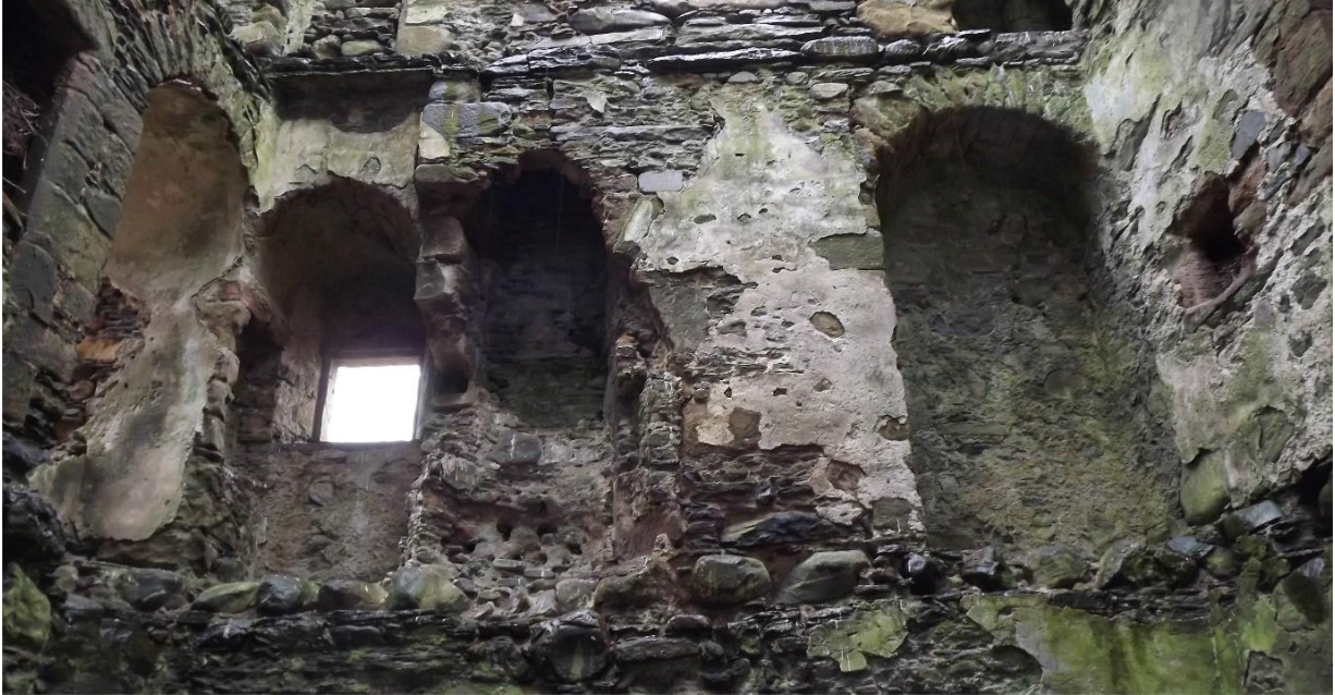
Occasional well-preserved areas of internal lime plaster survived, here at second floor level. These have been carefully incorporated into the new lime plaster where possible.
