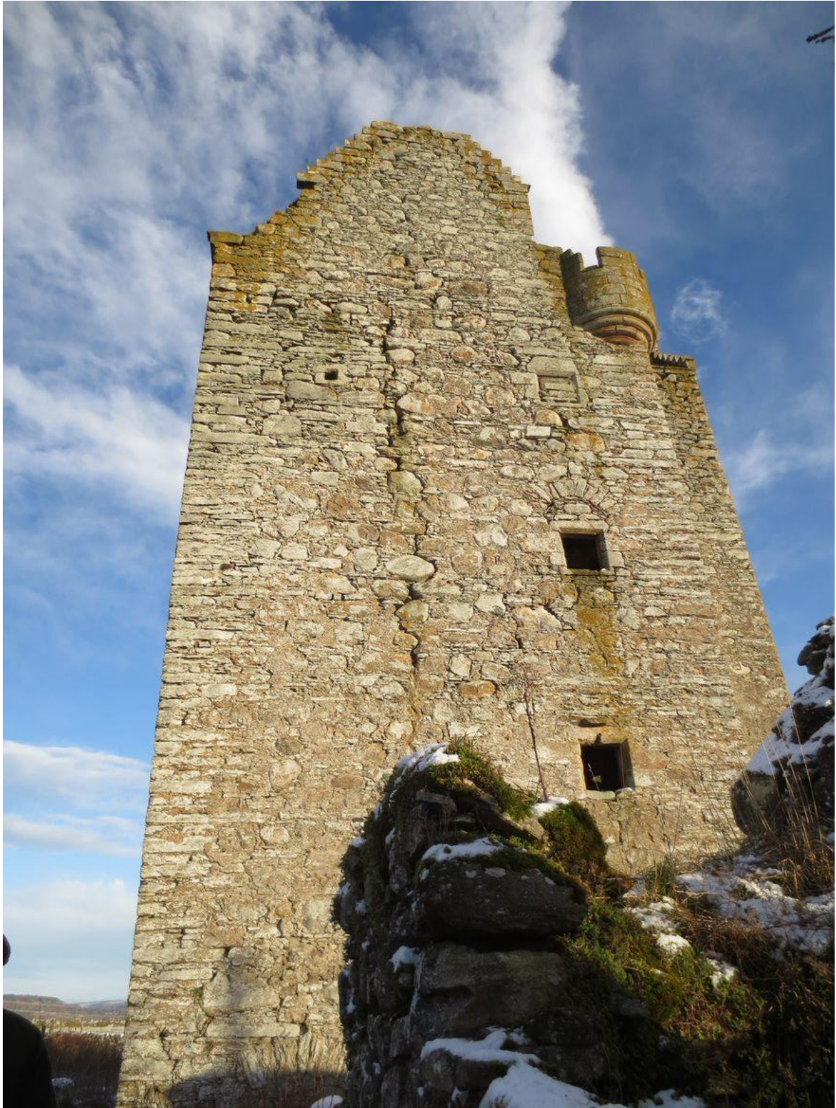
The main tower had serious cracking as well as the stair tower. The mixed quality of the rubble stone is apparent, as are some traces of the original render. Note too the window with the relieving arch, possibly used for materials access during construction.
