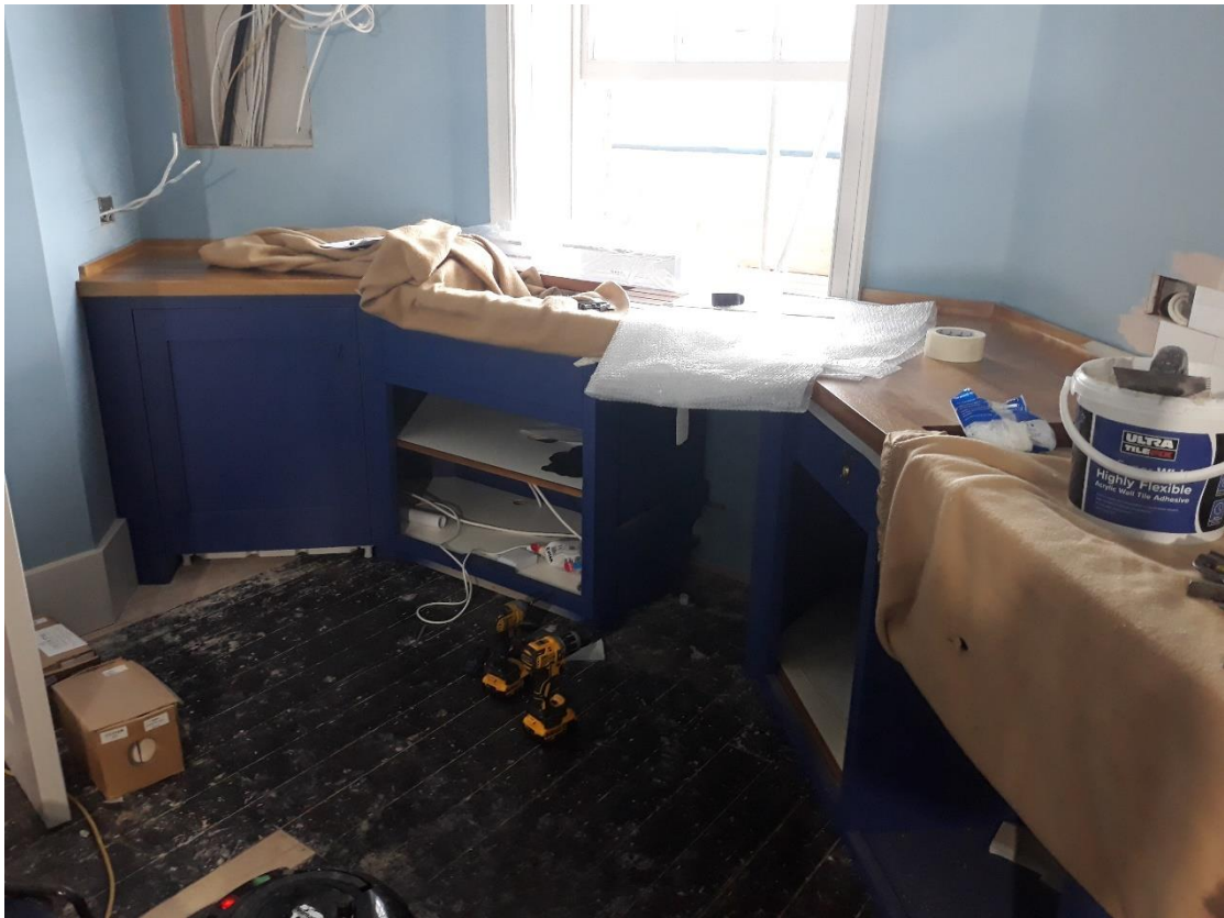
The kitchen under construction in Landmark's workshop at Honeybourne and during installation on the top floor.
