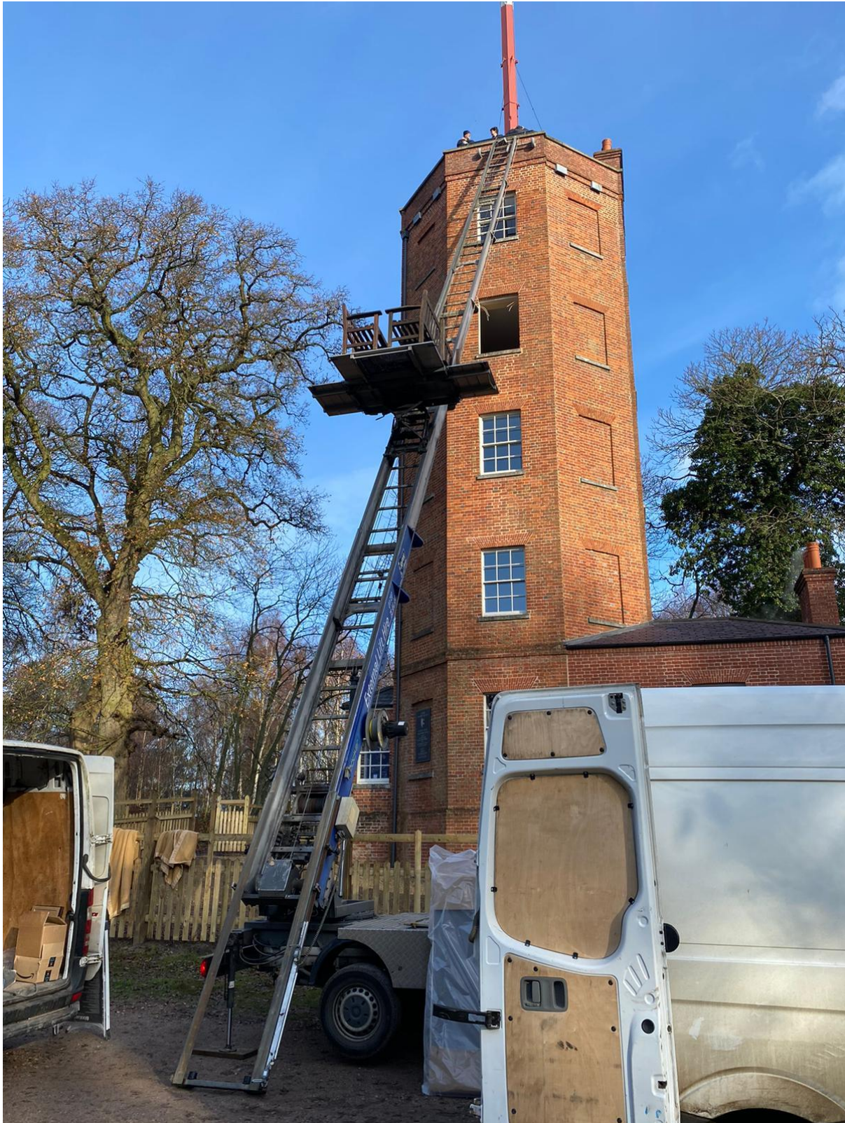
While Landmark's furnishings team have always relished a challenge (albeit with some gnashing of teeth) the Semaphore Tower saw a major innovation in the form of a furniture hoist, the only practicable solution here
