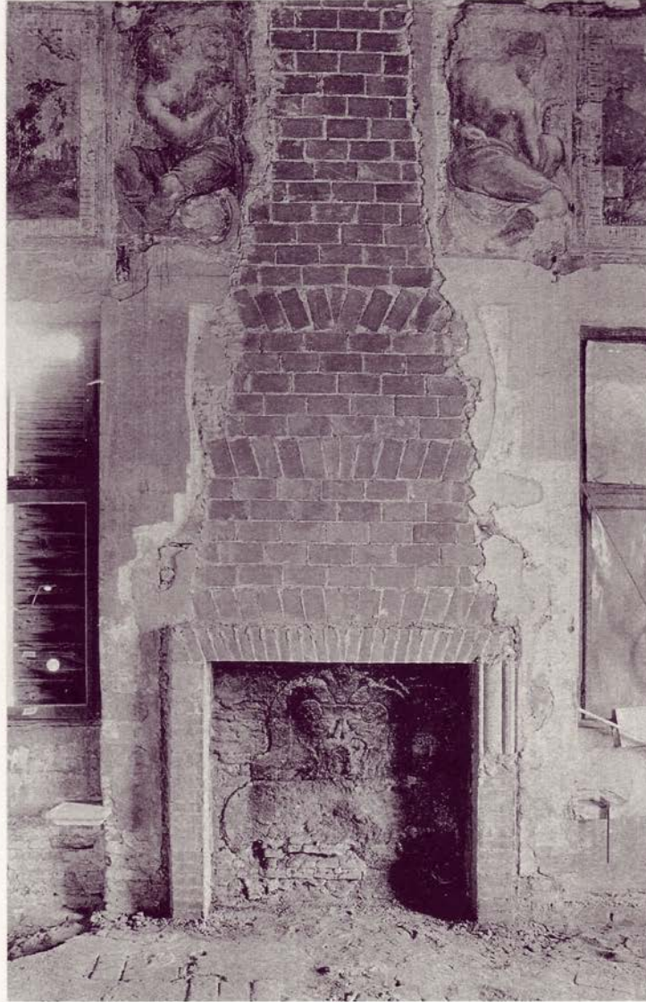
The 17 th century chimney piece in the stanza maggiore, emerging (left), and half way to reconstruction (above).
