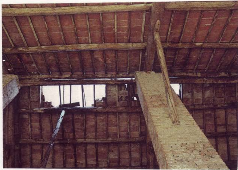
holes in the terra roof.
