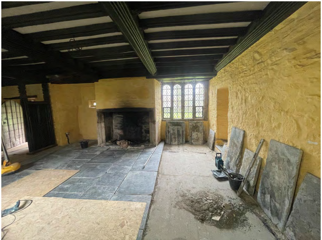
Once the underfloor heating mat was installed in the kitchen and great hall, the flagstones were carefully relaid.
