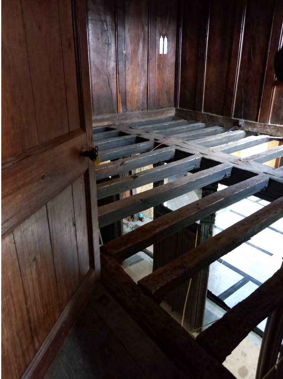
The floorboards were lifted throughout the first floor for asbestos removal and then rewiring. They were relaid with skilful splicing and patching in the few places damage had occurred.
