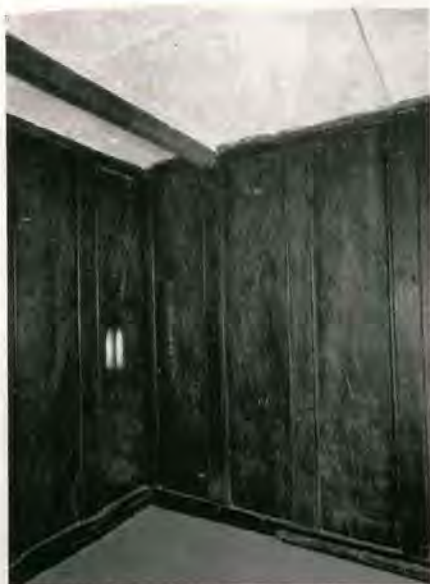
9.—POST-AND-PANEL PARTITIONING IN THE CLOSET WEST OF THE HALL CHAMBER, WITH A LITTLE WINDOW CUT IN ONE OF THE PANELS
