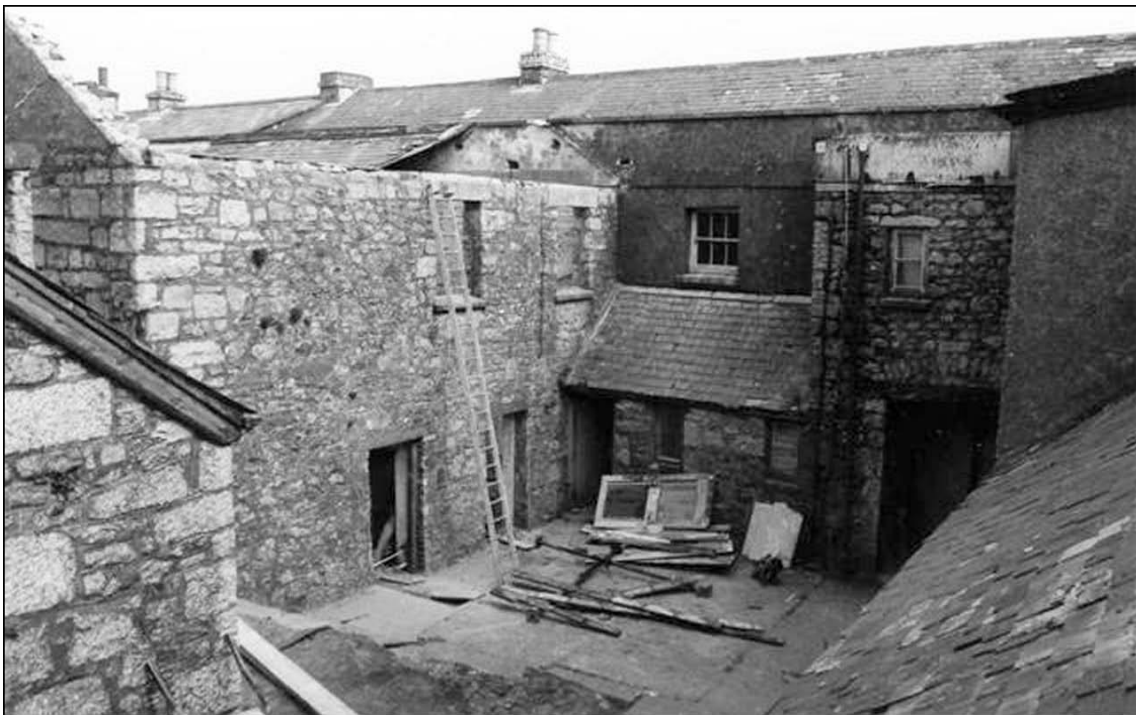
Starting demolition of the hotel outbuildings to create the courtyard. The gable end of the Radio Room is on the left and the sloping roof on the lower right was part of what is now Square Cottage
