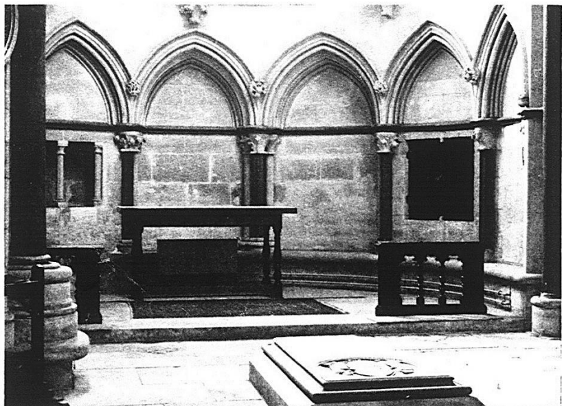
5.—THE CHAPEL OF SS PETER AND PAUL IN LINCOLN CATHEDRAL. Shafts and string courses are of Alwalton marble
