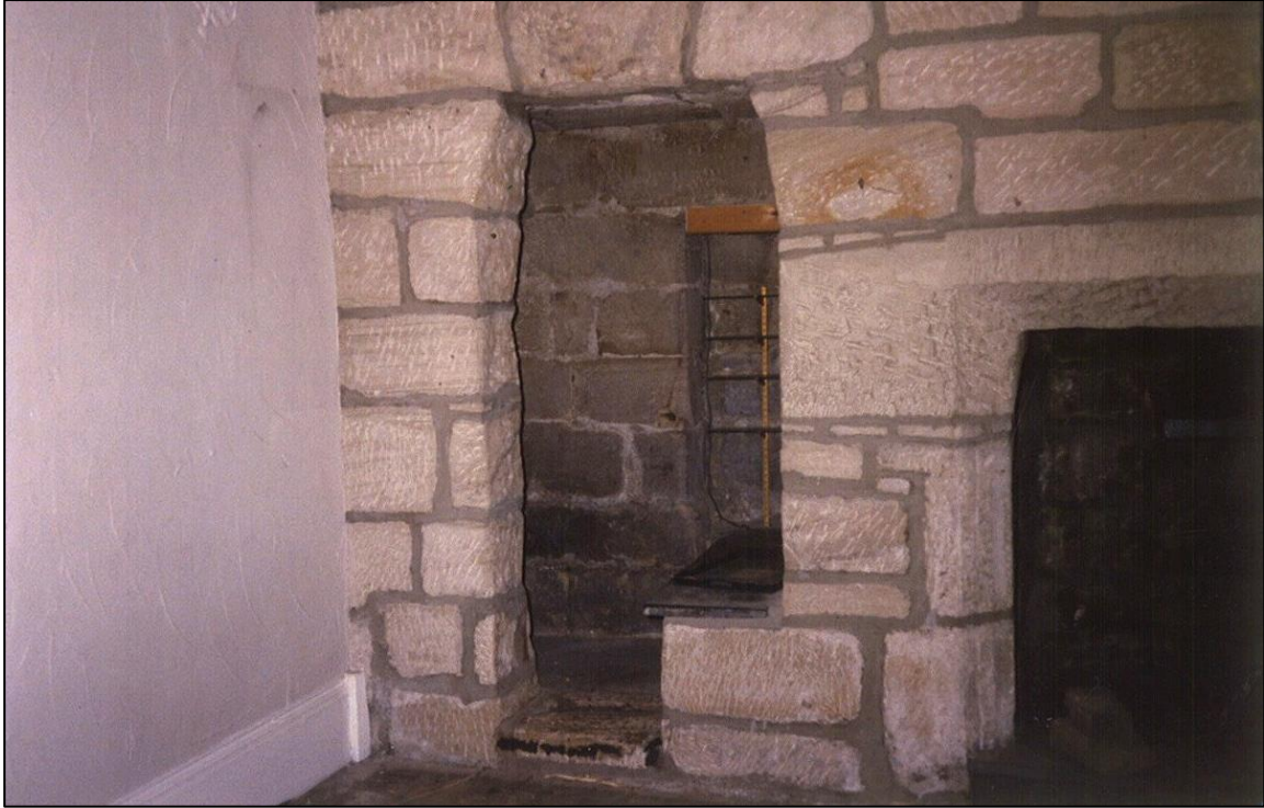
Opening made in 1960s into garderobe on north end of first floor, now built up.
