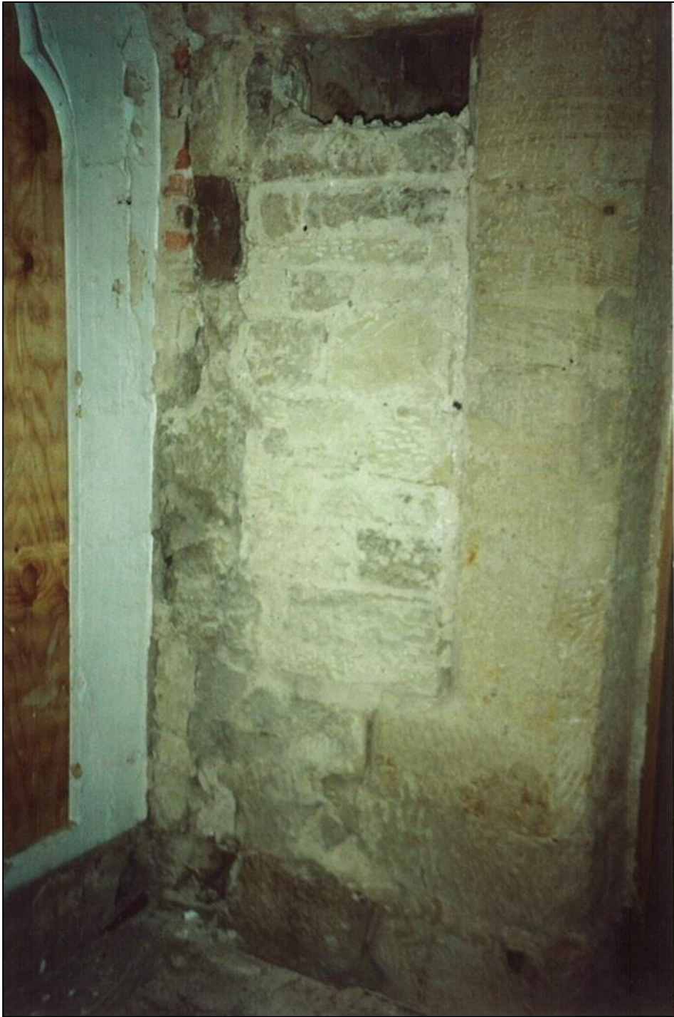
Discovering the original garderobe in the kitchen, to the right of the window.
