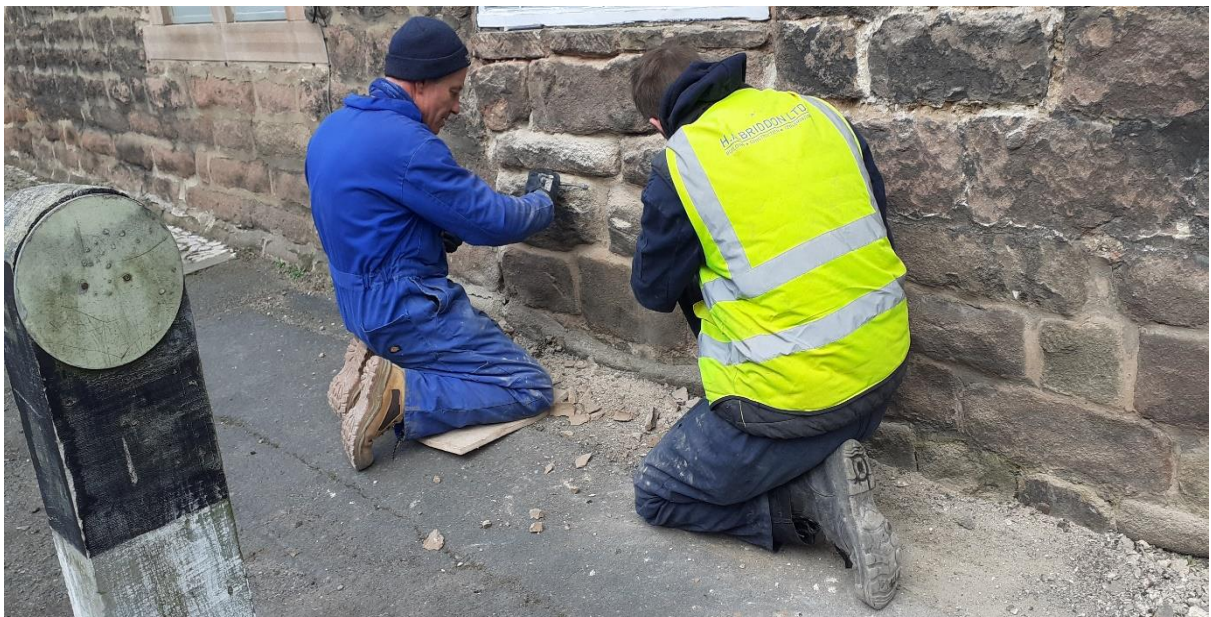
Apprentice Adam Winson worked alongside the experienced masons, gaining valuable experience, here raking out cement pointing with Ian Williams.
