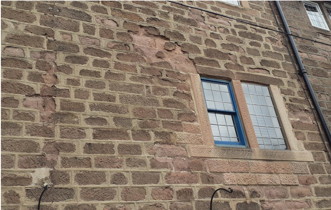
Above: masonry damage caused by clumsy re-pointing in cement.
