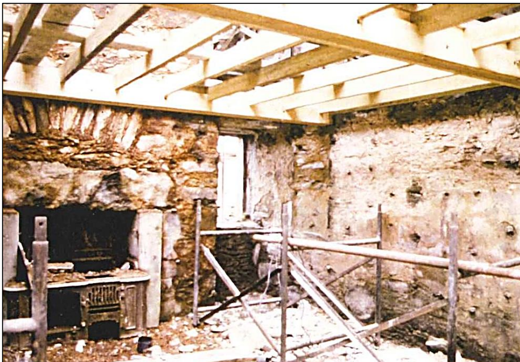
The big kitchen fireplace has a salt cupboard on the left, in which are all the treasures found during the repairs. The little jars and ink bottles were found in the attic in one of the blocked up windows.
