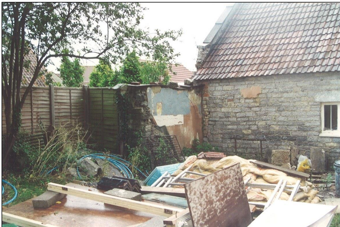
The roof was restored to its pre lean-to shape and the coping replaced.
