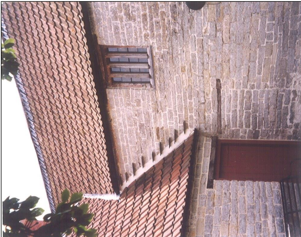
The door from the parish room into the old lean-to was blocked up
