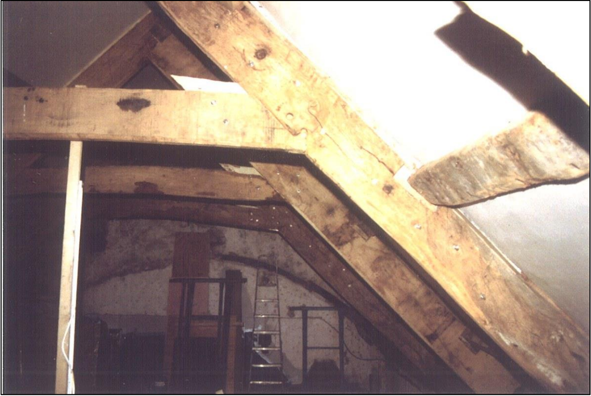
The roof of the north wing needed repairs.
