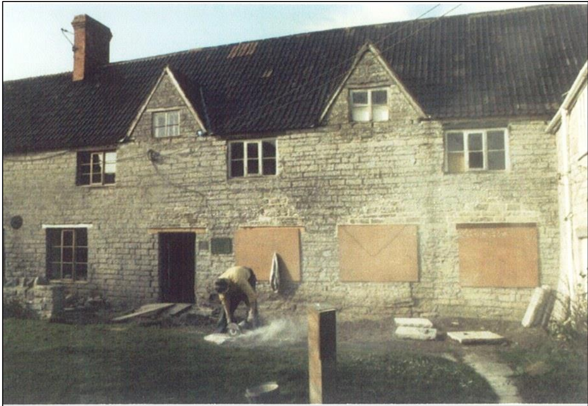
The windows on the ground and first floors were rotten and had to be replaced.
