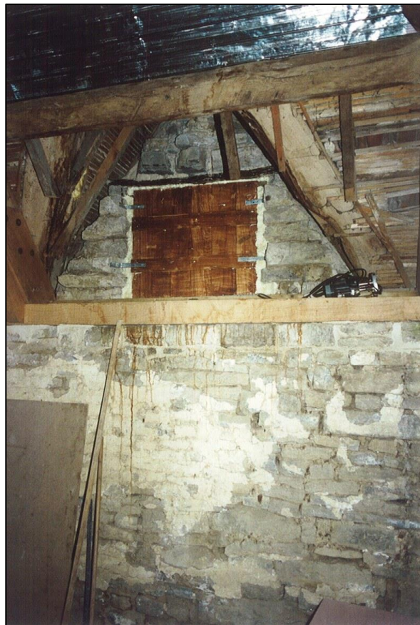
One of the blocked up dormers. The wall plate, damaged when the attic floor was put in, has been replaced.
