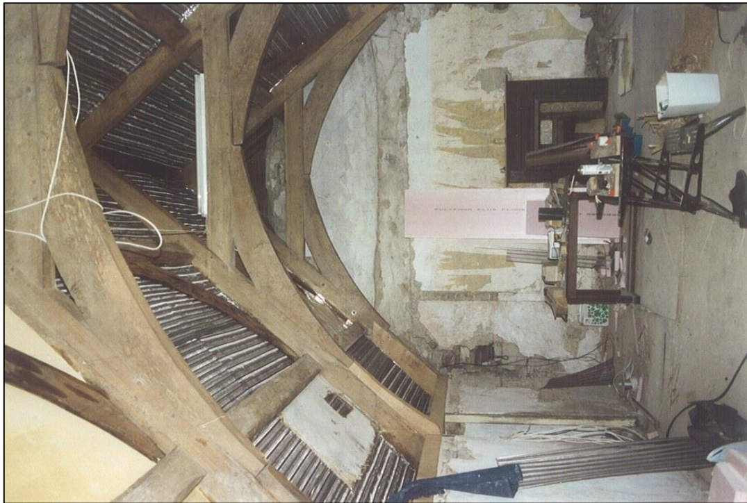
Looking east. Missing braces were restored, rotten and mutilated feet of the principal rafters were repaired and there were extensive repairs to the wall plates
