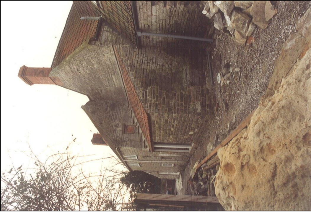
The new lean-to and on the far right the opening for the new front door is begun.
